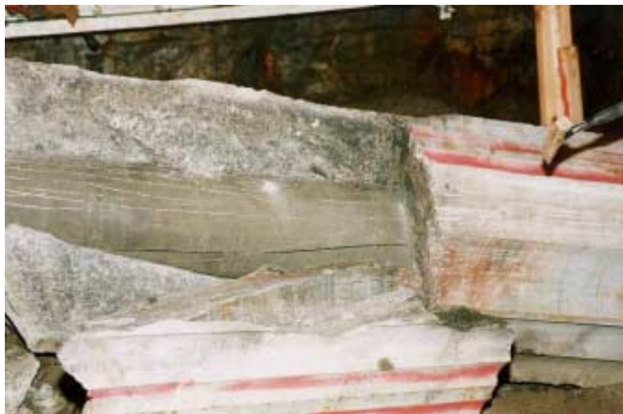
Figure 4-12 The first rock part has been removed from parcel S1 and the bentonite is partly exposed in the centre on the left side.
