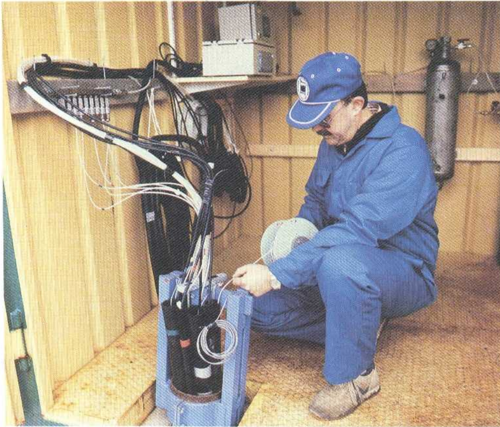
Figure 8.5 Top of monitoring hole, showing bundles of pressure tubings, signal cables etc. Calibration of pressure recording system by means of sounding in the stand-pipes.
