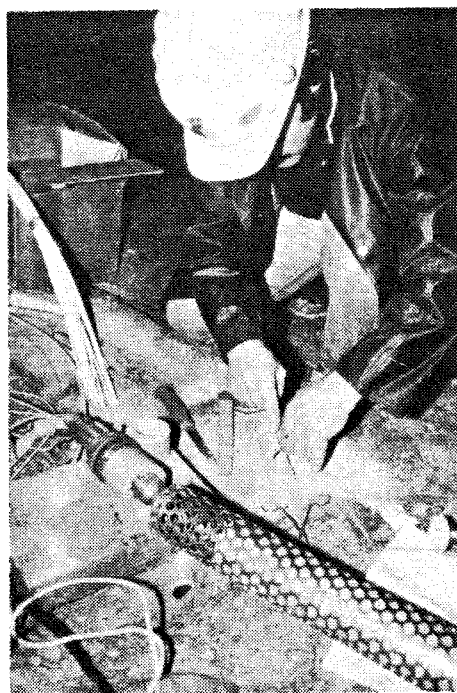
Figure 10-5. Highly compacted bentonite surrounded by a perforated copper tube used in the overlying backfill.
