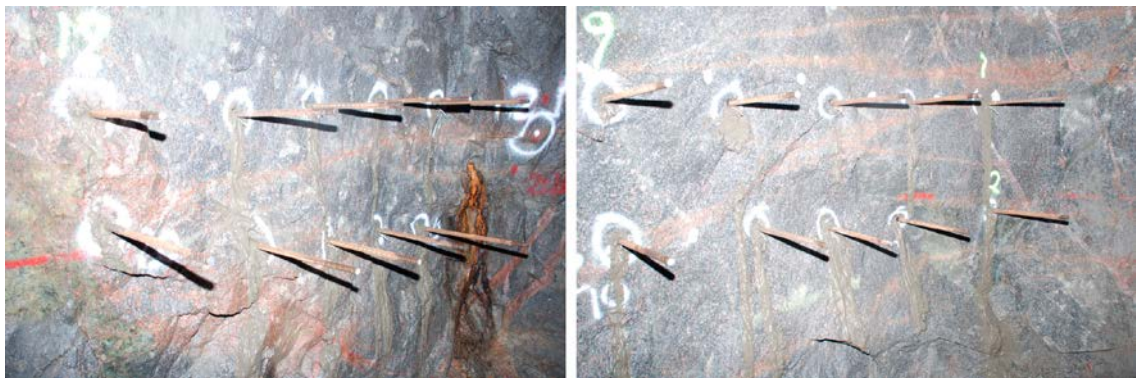
Figure 7-22. Setup of rock bolts at ÄSPÖ NASA 2376A ready to be tested.
