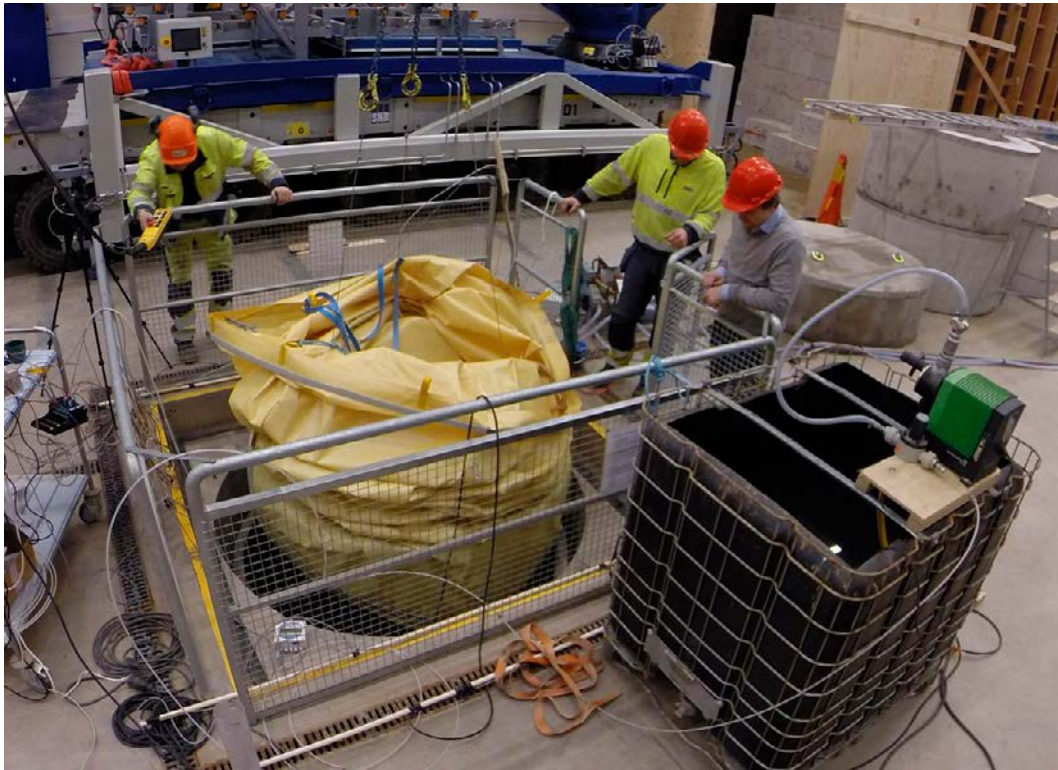
Figure 4-55. Photo taken when the assembled bottom plate and buffer protection sheet were lowered into the deposition hole in the Bentonite Laboratory at Äspö.
