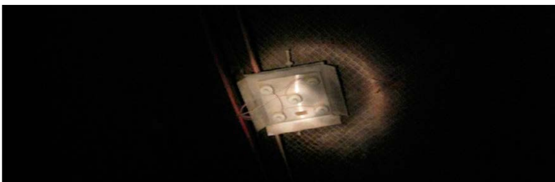
Figure 7-19. Smoke detector installed in the tunnel of Äspö HRL
