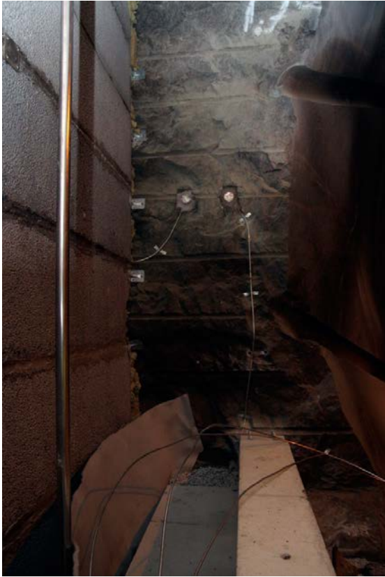
Figure 4-45. Detail photo showing (from left) filter of leca-beams and macadam, drainage (air) pipe, geotextile, bentonite seal of MX-80 (blocks and pellets) and concrete delimiters. All sensor cables are led in steel tubes.
