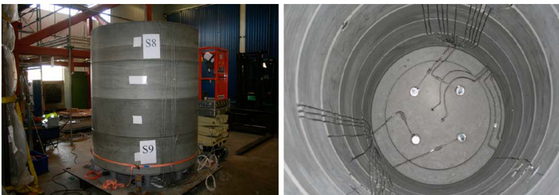
Figure 4-12. To the left ongoing assembly of a transition block with sensor sections and to the right a view inside the Supercontainer before the canister was placed, four pressure sensors are visible at the bottom.
