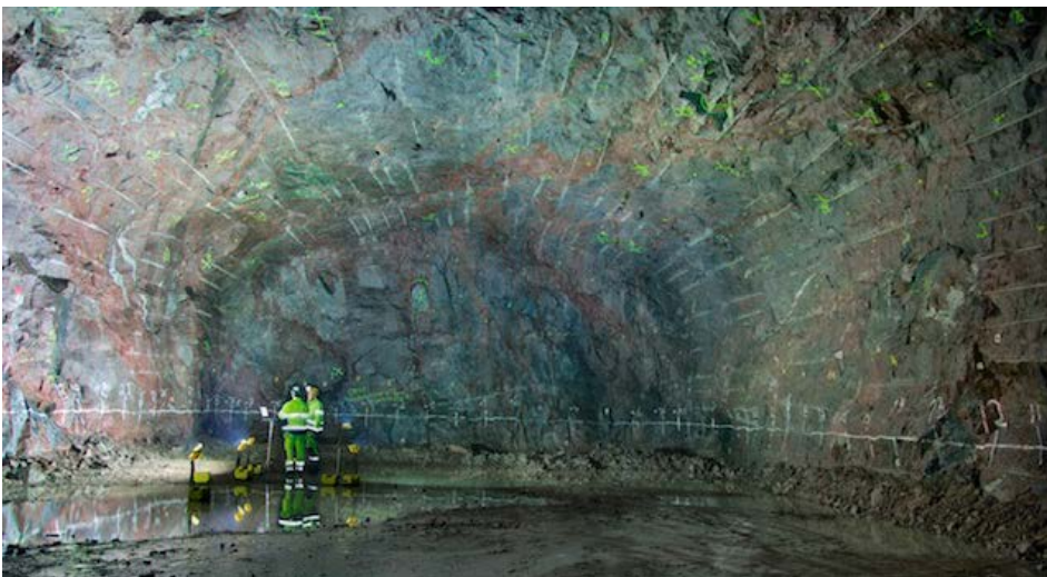
b) Photo of the completed niche located at the end of TASU that will be used for the KBS-3H experiments (TAS08).
