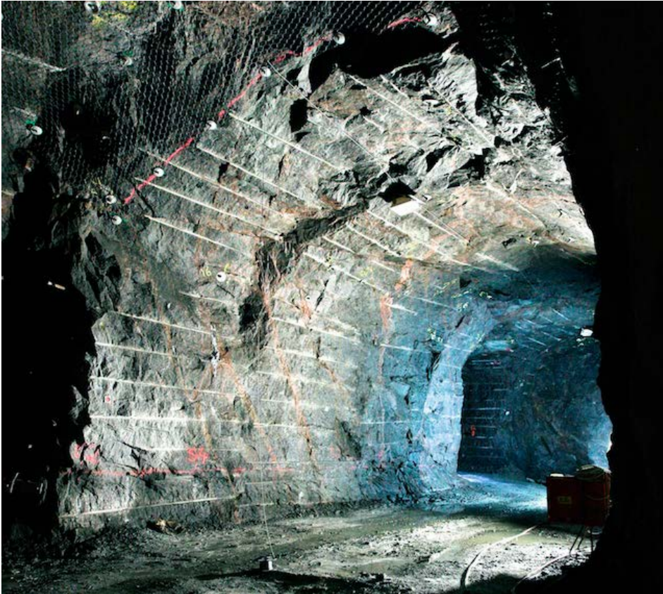
a) Example of the tunnel profile quality achieved in the TASU and TASP Tunnels.
