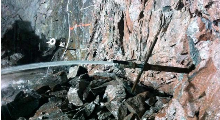
Figure 5-4. Example of a water flow encountered in a probe hole prior to grouting.
