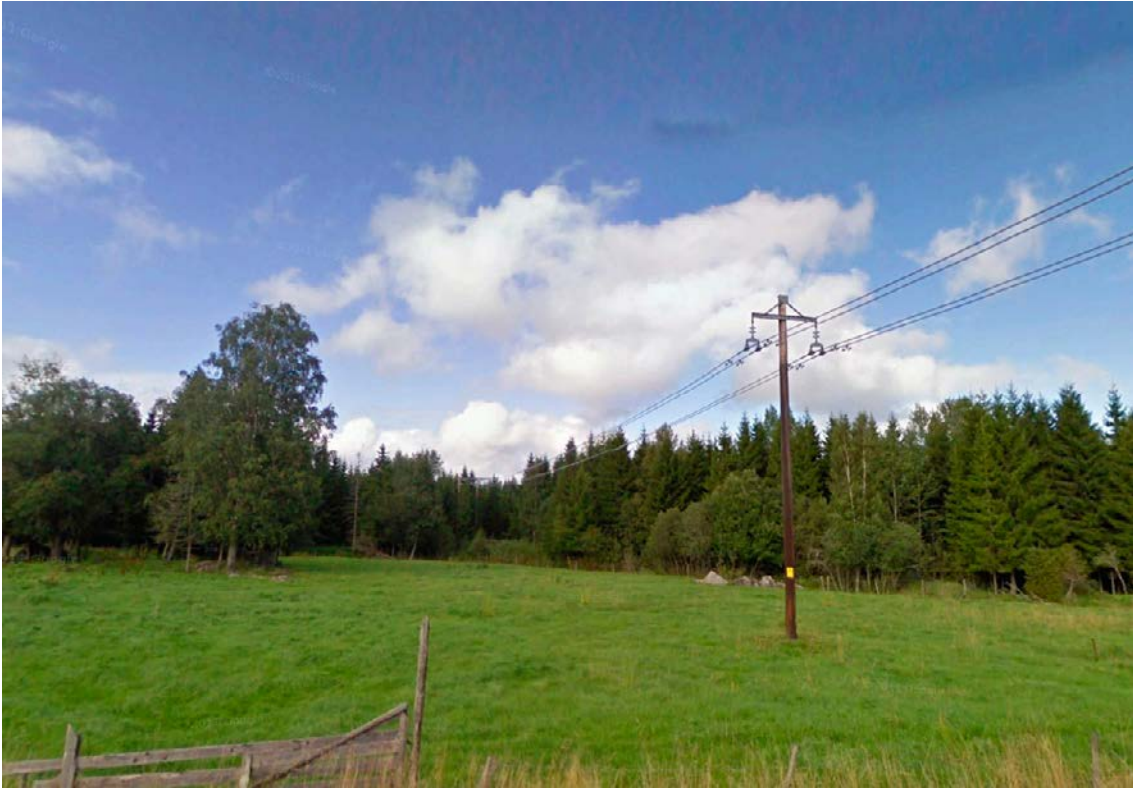
Figure 2-2. Photo of the DC overhead line between the inverter at Forsmark and the electrode at Fågelsundet. The voltage in the overhead line is of the order of magnitude 2 kV.
