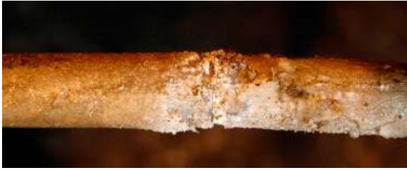
Figure 6-13. Attack in the joint between two rods, 1 cm outside the tunnel wall (KA3385A).
