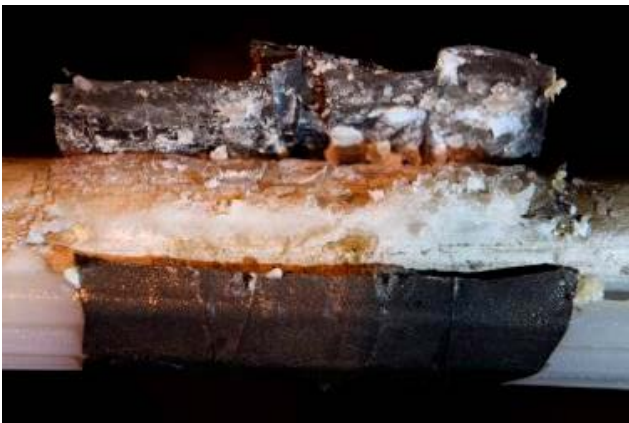
Figure 6-17. Severe corrosion under PVC-tape in the outer aerobic section (KA3385A, area 3, outside section 2).
