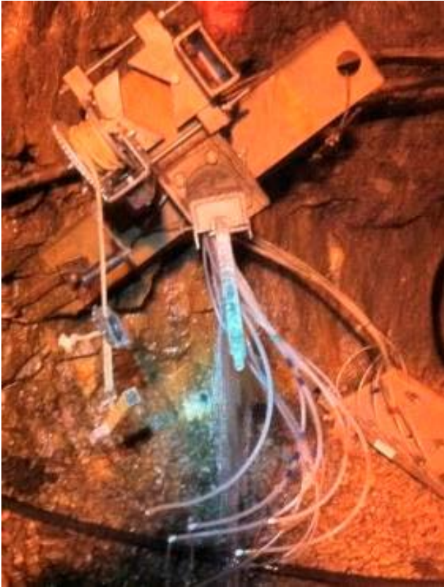
Figure 6-15. Severe corrosion on the whole surface of the first 2 m of rod (KA3105A) outside the borehole wall.
