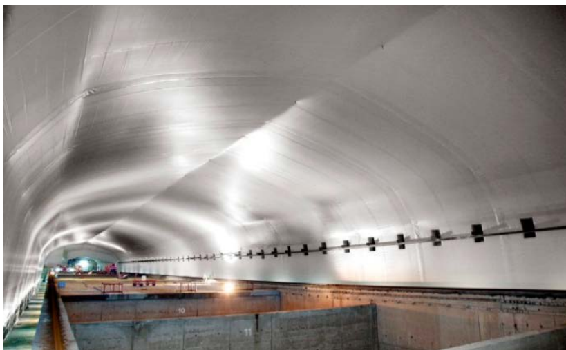
Figure 7-2. The tunnel cloth installed in 1BMA used to protect the concrete structure from groundwater dripping from the ceiling of the rock vault.
