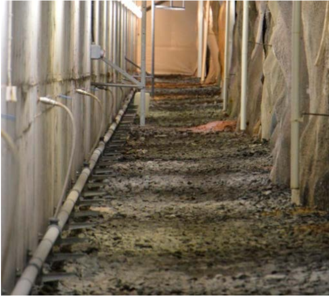
Figure 7-3. The drainage layer between the concrete structure in IBMA and the rock wall. This drainage layer also continues underneath the concrete structure.
