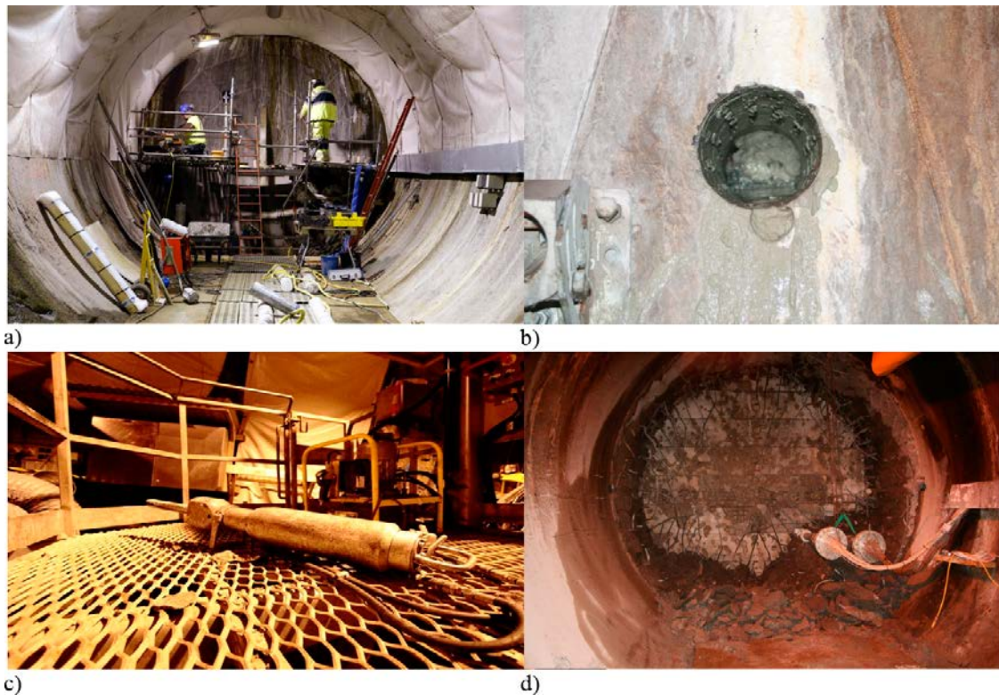
Figure 2-7. a) The drilling machines placed on the rig. b) Backfill material squeezed out through a drilled hole in the concrete plug. c) The hydraulic breaker used at the demolition of the plug. d) Remaining of the concrete plug and its reinforcements together with the retaining wall. The cables placed in tubes passing through the plug are visible on the right side.
