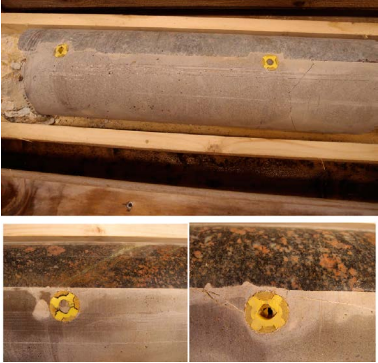
Figure 2-6. Close up pictures of the cores taken from the interface between the concrete plug and the rock. The yellow grouting tubes are embedded in grout.
