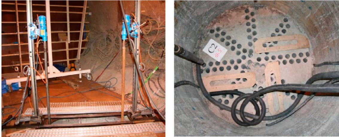
Figure 4-1. a) The core drilling machines standing on the tunnel floor. b) Holes from cores taken from a buffer block. Wooden templates were used to position the drill bit.
