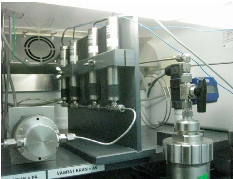
Figure 2-12. Two pairs of pressure-resistant redox electrodes installed on-line on the circulating groundwater in one of the stainless steel circulation systems.
