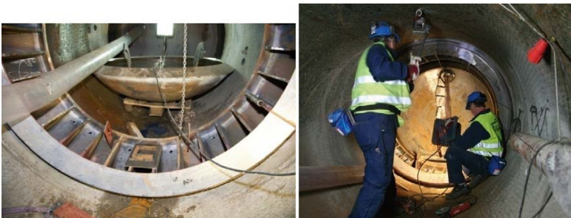
Figure 4-33. Installation of the compartment plug collar and cap. The cap was raised using a hand winch.
