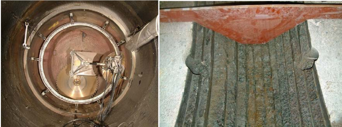
Figure 4-31. The rock notch was excavated with parallel-cut sawing. Several cuts were made and the slabs broken away creating a notch. The method proved to be functional. The left image shows the saw mounted in the drift, the resulting notch profile is shown to the right.
