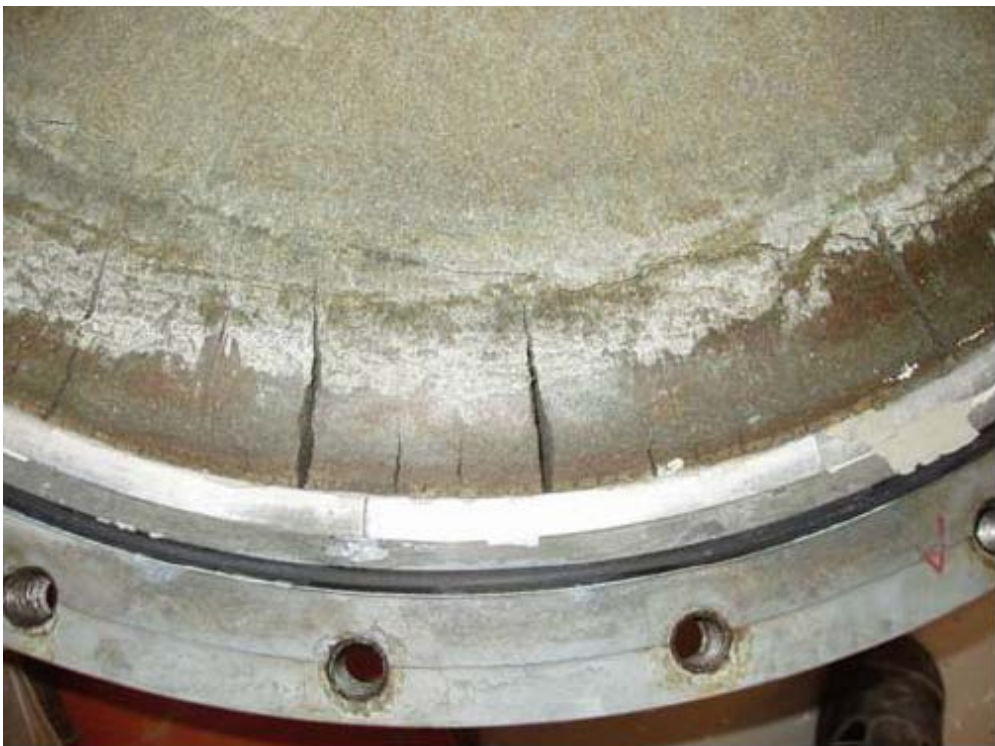
Figure 5-57. Close-up showing some of the radial cracks.
