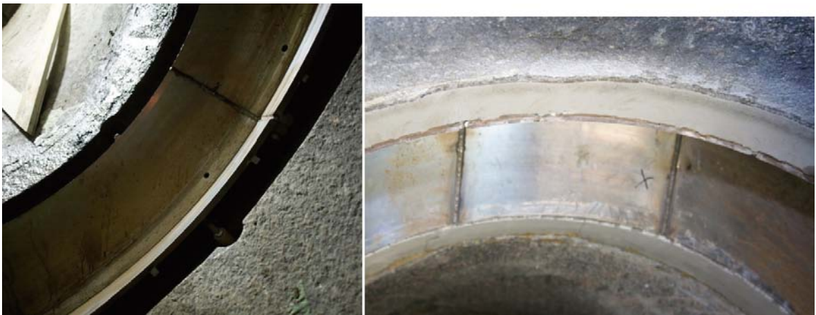
Figure 4-32. Fastening ring positioned in the rock notch to the left. The right image shows the top of the completed fastening ring casting.
