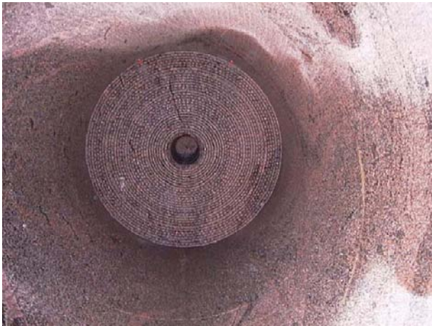
Figure 9-5. The end of the 95 m drift at the Äspö HRL showing the final shape of the face and occasional grooves.
