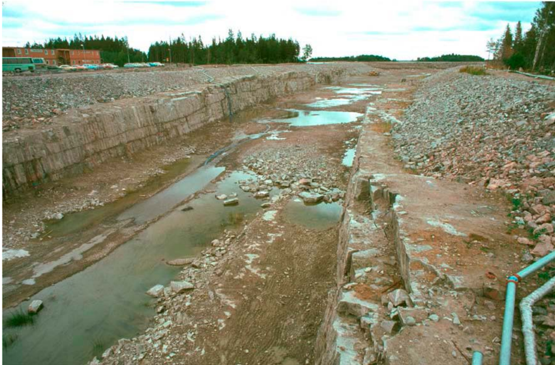
Figure 5-37. Photograph of the inlet water channel at Forsmark (Follin et al. 2007b).
