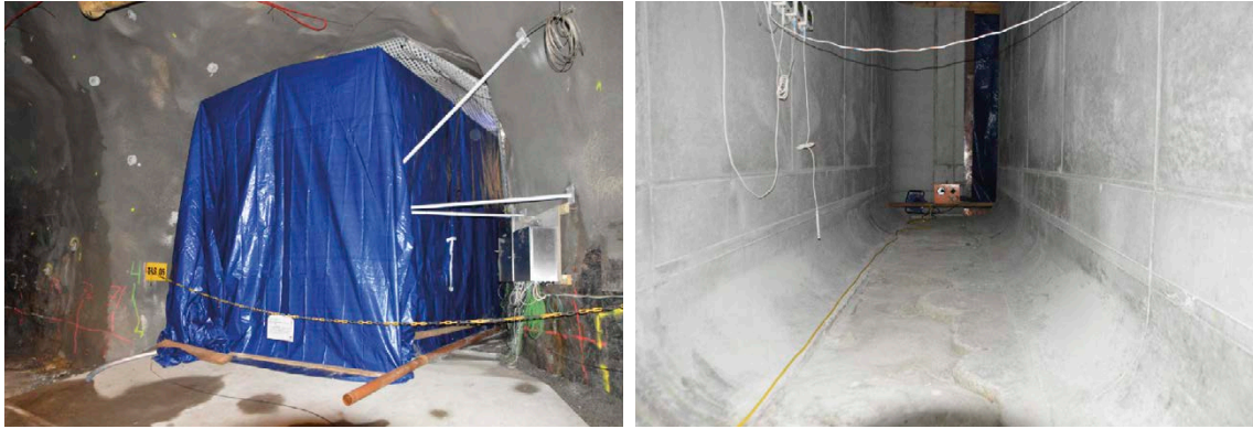
Figure 6-6. The concrete structure was covered with a tarpaulin to protect in from the wet atmosphere in the tunnel and dripping groundwater (left image) and dried for a few months using two dehumidifiers (right image). One of the dehumidifiers (orange box) is seen in the centre of the image. (Mårtensson and Vogt 2019).
