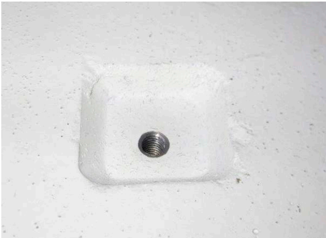
Figure 6-7. The hole in the concrete tank used in the tests reported by Lundqvist. 1
