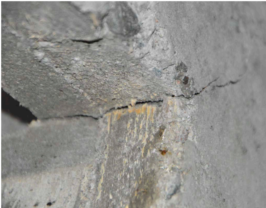
Figure 6-4. Penetrating crack in the upper corner of a doorway between two adjacent waste compartments.
