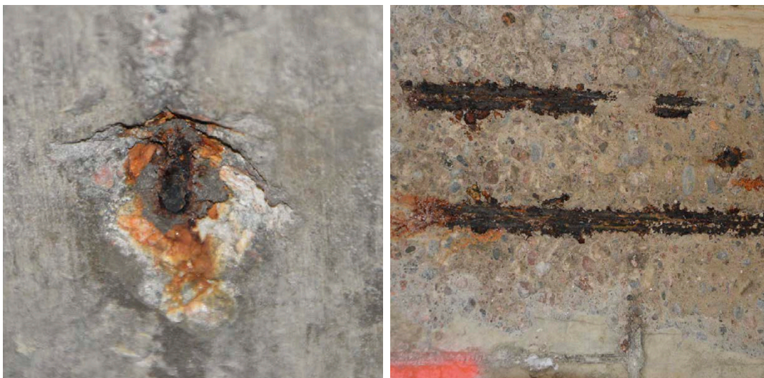
Figure 2-15. Corrosion of a steel tie rod (left image) and spalling of the concrete covering layer due to corrosion of the reinforcement bars (right image).
