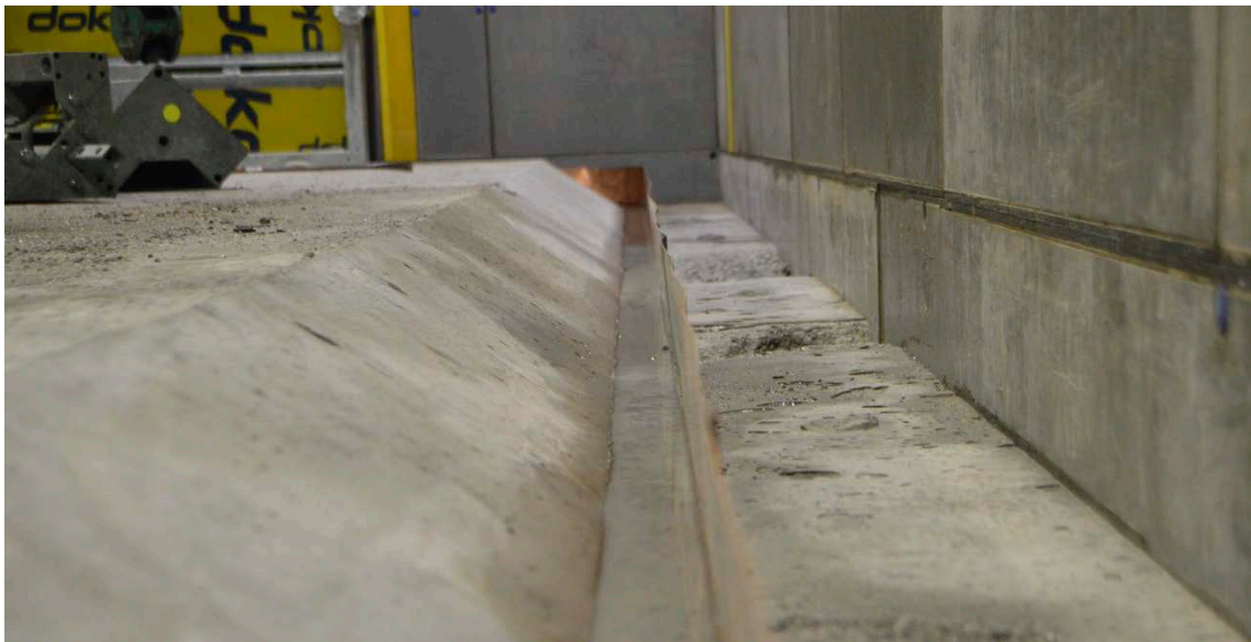
Figure 2-19. The image shows the recess in the peripheral part of the slab (i.e. the future position of the outer walls) of the concrete caisson that constituted the final part of the development programme and which was constructed at the Äspö Hard Rock Laboratory (Mårtensson and Vogt 2020). The recess improves the mechanical strength of this joint and the visible copper joint seal in the left part of the recess contributes to a low hydraulic conductivity of the joint.
