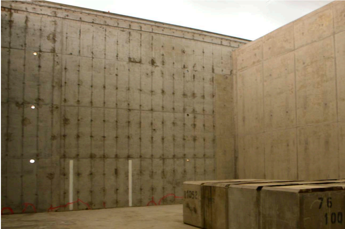
Figure 2-12. The interior of one of the compartments in IBMA showing the holes in the existing outer walls which were planned to be used for grouting of the waste packages at closure of the repository. The dark spots show the position of the tie rods used to keep the formwork together during casting.
