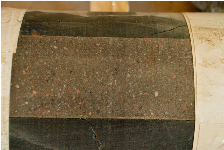
Figure 6-9. A part of the core, without signs of separation, made of standard concrete for casting under water extracted from a depth of about 220 meters (Mårtensson 2019).
