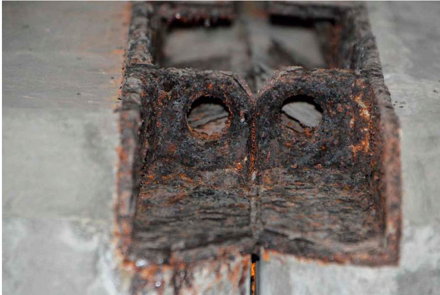
Figure 6-5. The lifting eye in the upper parts of a concrete mould with obvious signs of severe corrosion. The concrete mould has been stored in an open compartment for many years and is thus not representative for all concrete moulds in IBMA.
