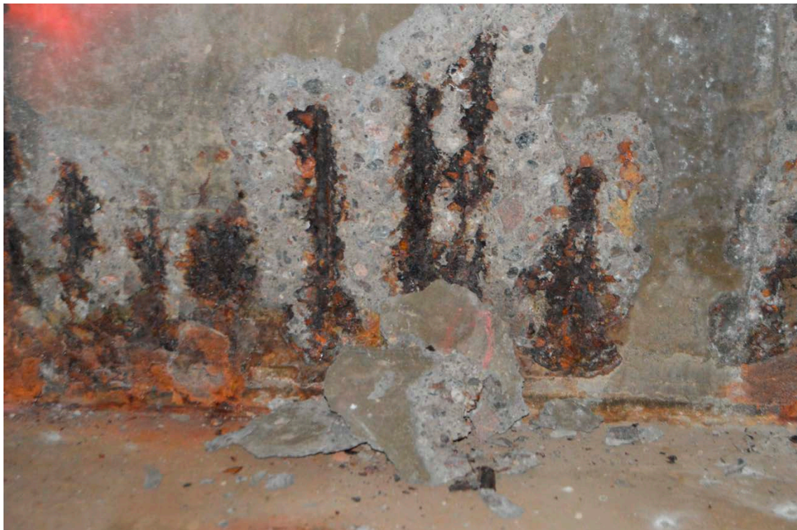
Figure 4-9. Concrete spalling due to corrosion of reinforcement bars on the inside of the existing outer walls of the concrete structure in IBMA..
