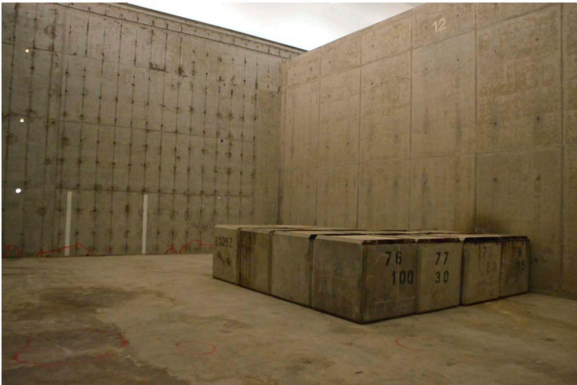
Figure 6-3. The interior of compartment 12 in IBMA showing the inner wall to the right and the existing outer wall to the left as well as some concrete moulds. Note the holes in the existing outer walls in the left part of the image planned for use during the now abandoned grouting of the waste packages.
