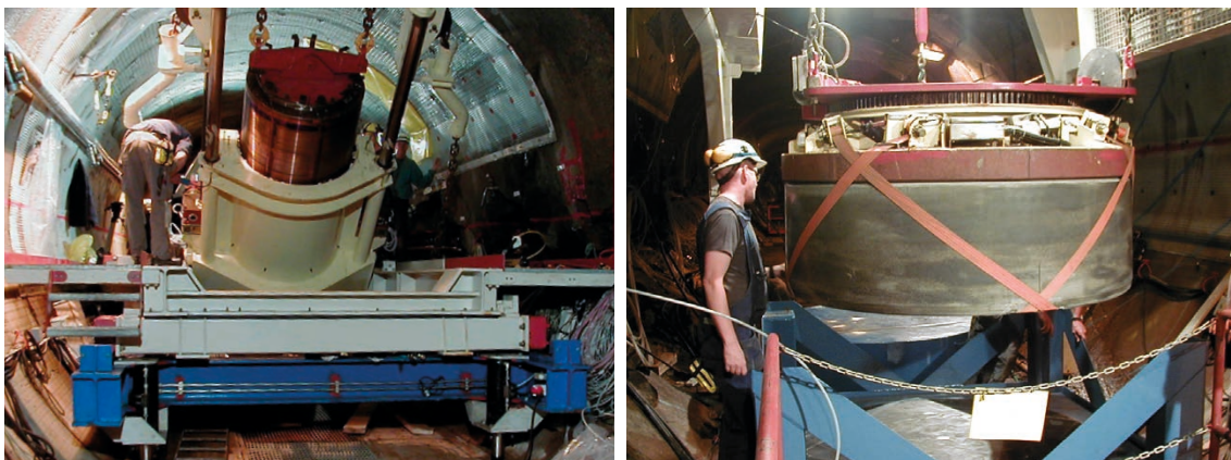
Figure 4-1. Photos from the installation of the prototype repository in the early 2000s. On the left, a canister placed in a deposition hole. On the right, a buffer block to be placed in a deposition hole.
