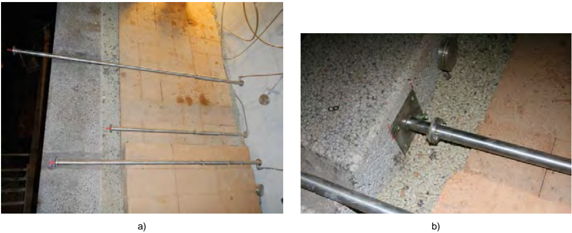
Figure 6-8. Parallel installation of bentonite backfill blocks, pellets and LECA beams. In the photos, the installed displacement sensors are also shown together with some of the total pressure sensors.
