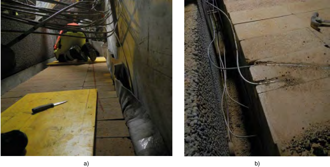
Figure 6-7. Photos showing the installation process of bentonite backfill between the concrete back-wall and the LECA beams.
