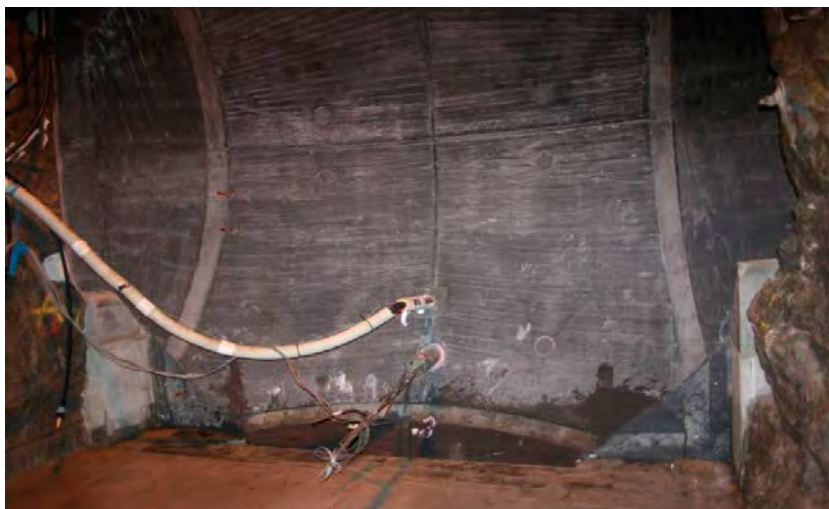
Figure 7-11. Lead-through in the concrete dome. The upper is for cables of measurement equipment installed inside the concrete dome and the bottom is for equipment installed in the bentonite seal and in the slot (i.e. not those cast inside the concrete dome).
