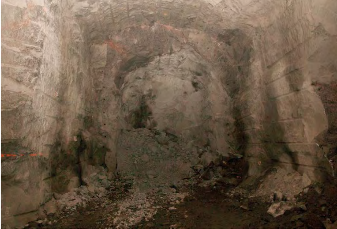
Figure 3-5. Photo of the test tunnel TAS01 during ongoing excavation of the third round. The perimeter boreholes to be used for separate charging and blasting of the peripheral tunnel contour are visible.
