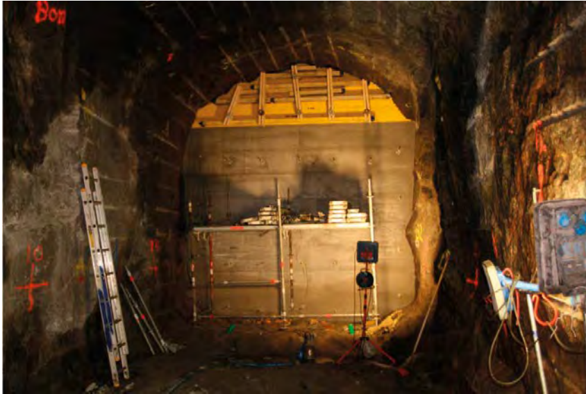
Figure 6-2. Photo of the concrete wall during removal of the formwork subsequent to casting.
