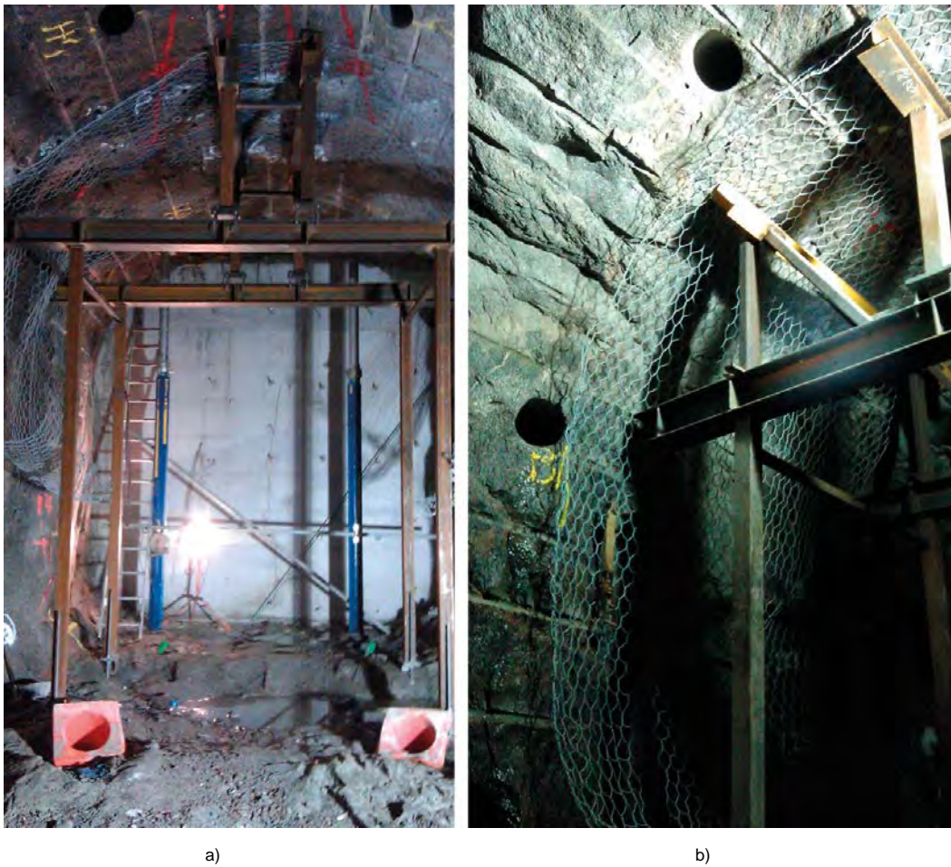
Figure 3-9. a) Photo of the erected safety scaffolding including a tunnel mesh to protect workers from falling rocks b) Detail of the scaffolding with two of the \varnothing 250 mm boreholes visible.
