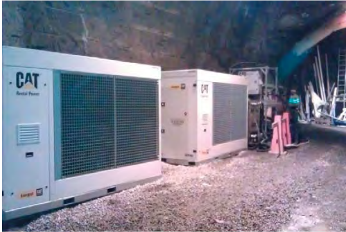
Figure 6-22. The two cooling machines placed in the main tunnel TASJ.
