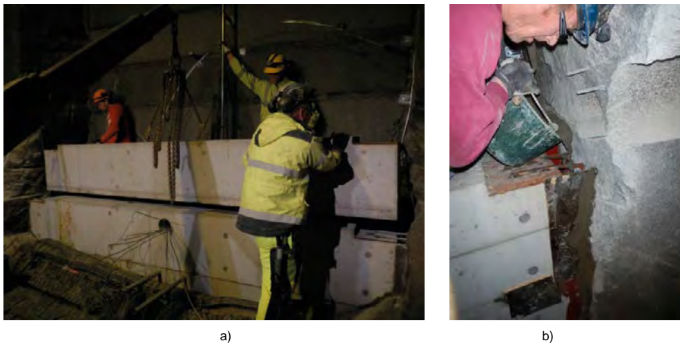
Figure 6-17. Installation of a concrete beam, a) lifting it into place, b) filling of gap between beam end and the rock wall.
