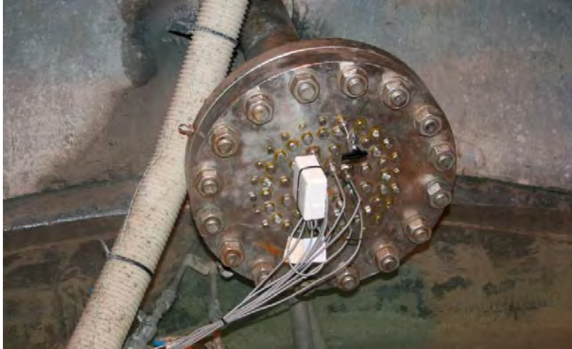
Figure 7-12. Lead-through in the concrete dome, intended for cables of measurement equipment installed in the bentonite seal and in the slot (i.e. not those cast inside the concrete dome). Here also shown with the water tight connection.
