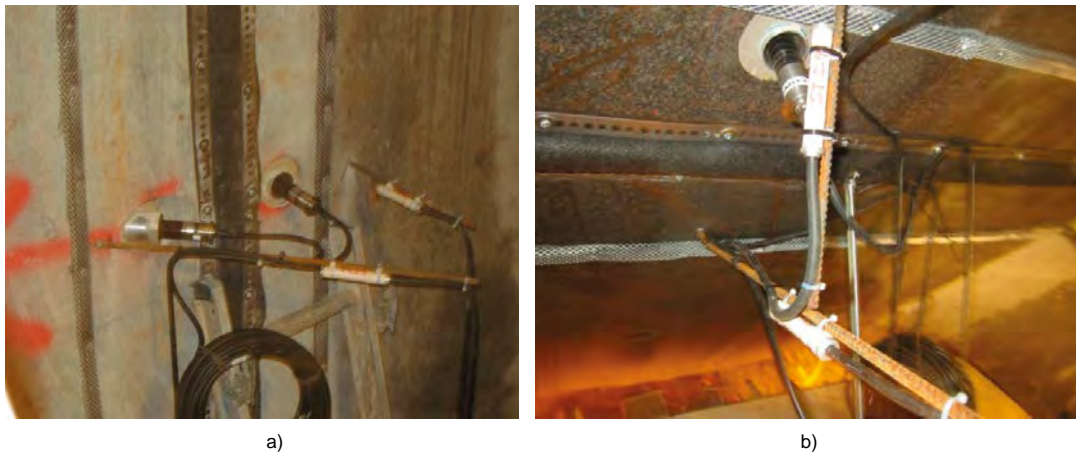
Figure 9-42. Photo of the two strain gauges ST23, (Figure (a)) and ST25 (Figure (b)) that failed during contact grouting.
