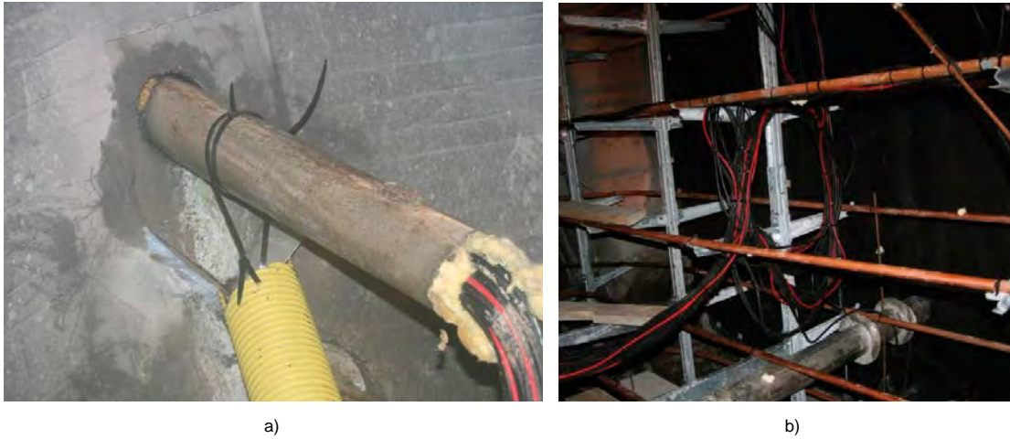
Figure 9-53. Located leakage through the cable bundle for sensors installed in the concrete dome.
