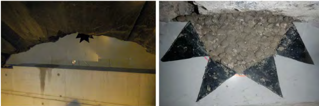
Figure 6-34. Left: Photo showing the steel plate fastened against the uppermost row of bentonite blocks Right: Close-up showing the opening through which the last pellets were installed.
