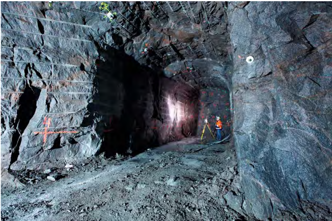
Figure 3-6. Photo of the completed test tunnel TAS01. Geodetic survey is ongoing to mark out positions of the plug components.
