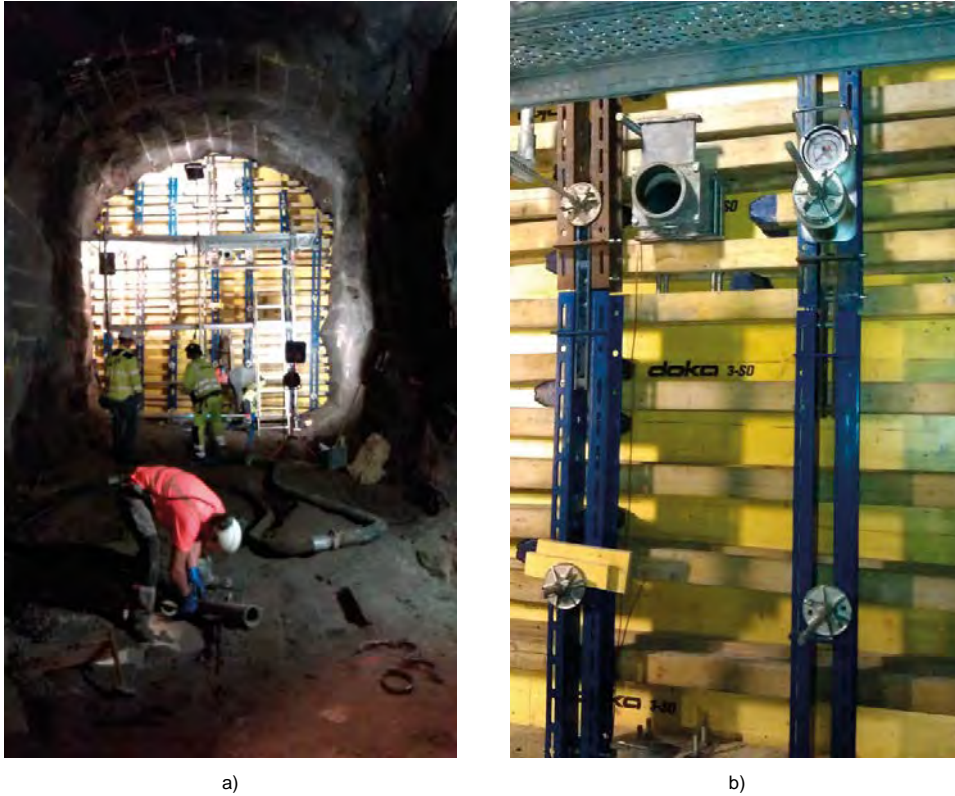
Figure 6-4. a) Complete formwork for the concrete back-wall. b) Formwork detail including analogue pressure gauge.
