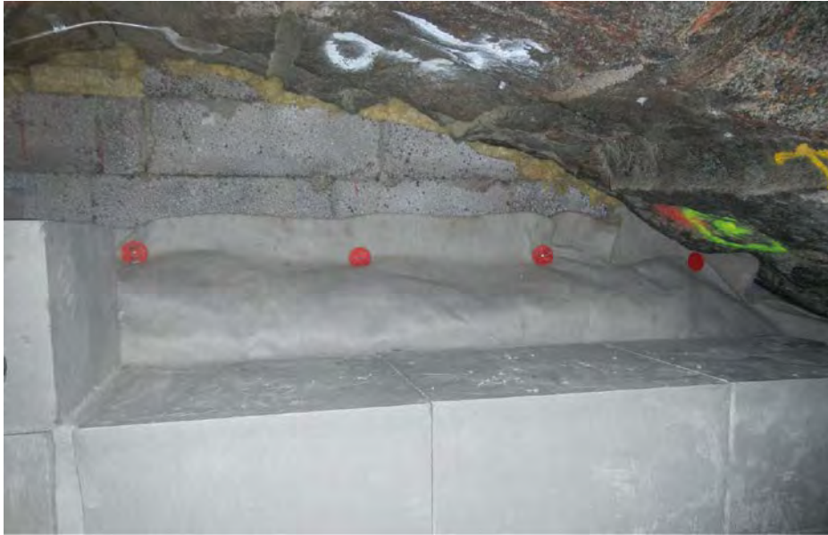
Figure 6-32. Photo showing the space left above the gravel section. The geotextile was folded in over the uppermost gravel surface.
