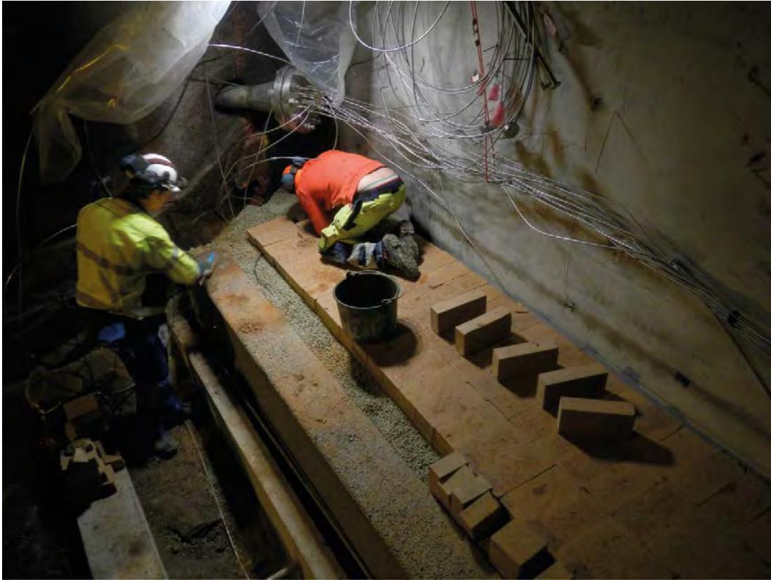
Figure 6-5. View of the arrangement of bentonite blocks and pellets in the backfill transition zone for DOMPLU.
