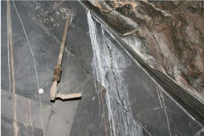
Figure 9-50. Observed water leakage in the interface between the concrete dome and the rock, in the top of the slot (at 13 o'clock). Note that the dark line on the face of the dome is water not a crack in concrete.
