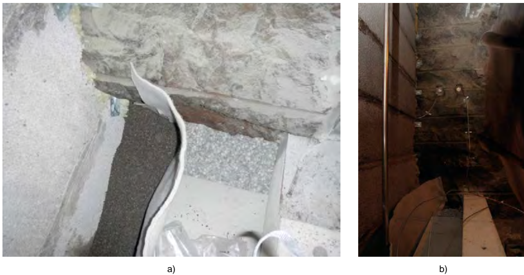
Figure 6-12. a) Simultaneous installation of gravel filter (macadam 2–4 mm), middle delimiter (geotextile), bentonite seal (blocks and pellets) and outer delimiter (concrete beams). b) Side-view of the drainage pipe used for de-airing, ending near the tunnel roof inside the gravel filter. The other drainage pipe ends at the bottom of the gravel filter (not visible in the photos).
