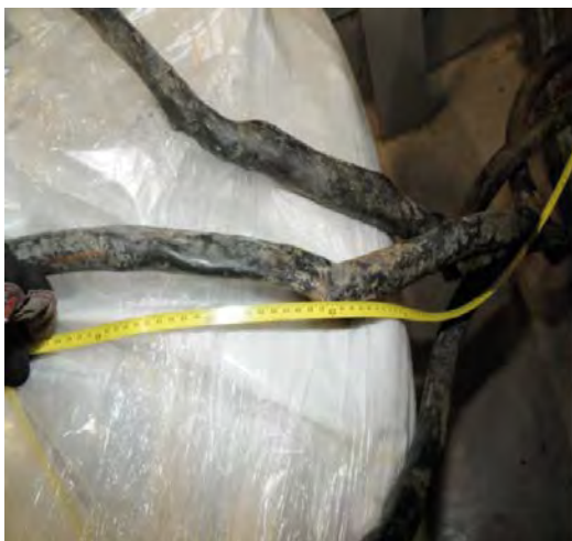
Deformed cable from canister in deposition hole No 6.
