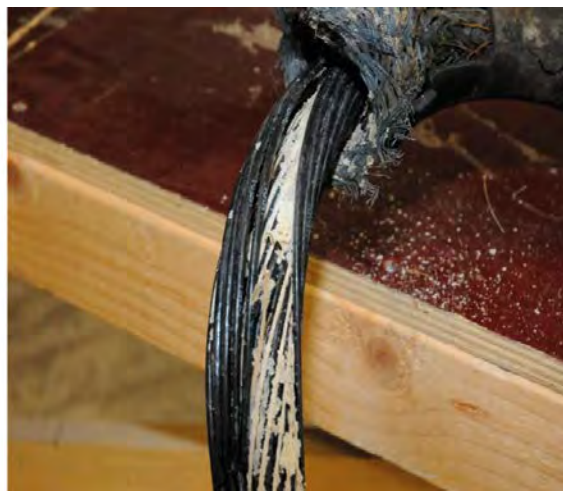
Stripped cable from canister in deposition hole No 6 with exposed wires.
