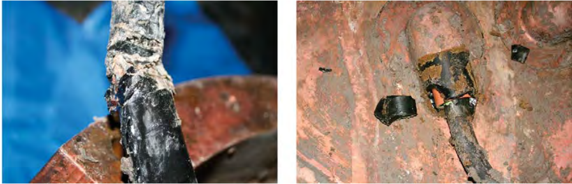
Figure 4-18. Left: Damages observed close to the periphery of the canister. Right: Damages observed where the cables were going through the lower canister lid. (Figure 4-8 in Johannesson and Hagman 2013.)
