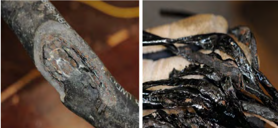
Drill damage on cable from canister in deposition hole No 6.
