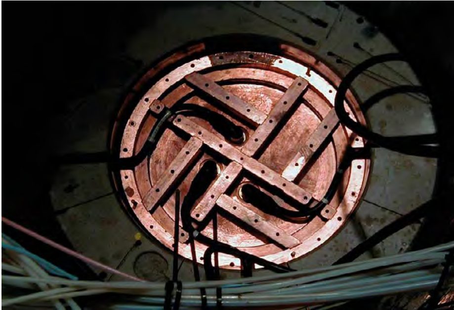
Figure 2-12. Connection of power supply cables to the canister lid. Supporting bars were mounted and on top of them a second lid in order to avoid any major swelling pressure on the cables.
