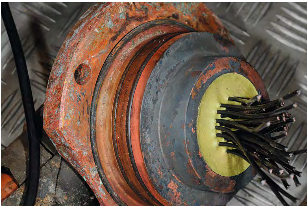
Figure 5-48. "Nose" for electrical wire penetrations. Corrosion products were found only inside the first O-ring.
