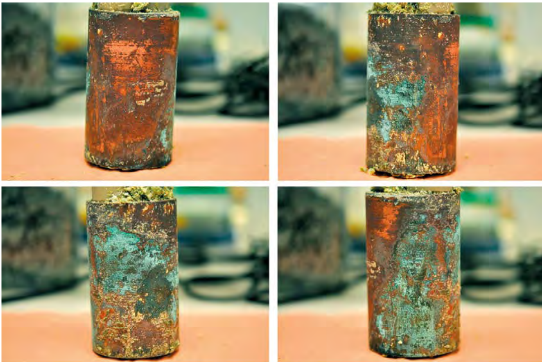
Figure 5-45. Appearance of copper electrode “Black” immediately after removal from the bentonite block. The top pictures show the two sample areas termed “H” (left) and “V” (right) in Figure 5-43. (Figure 3-2 in Rosborg 2013b.)
