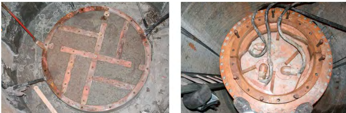
Figure 4-12. Left: After removal of the upper lid. Right: After removal of the bentonite/sand mixture and uncovering of the cables and their connections on the lower canister lid. (Figure 4-7 in Johannesson and Hagman 2013.)
