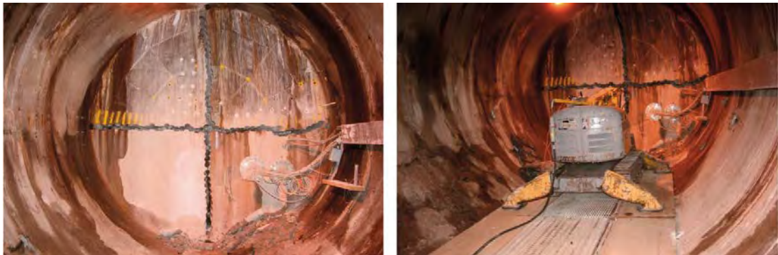
Figure 4-4. Left: The cross-like pattern of the core drilled holes through the plug. Right: The machine used for demolition of the concrete plug. (Figure 2-2 in Johannesson and Hagman 2013.)
