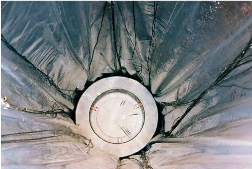
Figure 2-15. Buffer protection sheet seen from above. The bottom bentonite cylinder and the first ring have already been emplaced. (Figure 1-3 in Wimelius and Pusch 2008.)
