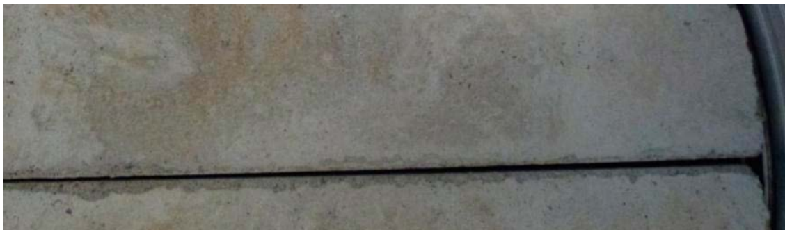
Figure 4-50. The gaps between the concrete beams in Test 5 were considerably larger than in previous tests. The largest voids were about 1–2 mm.
