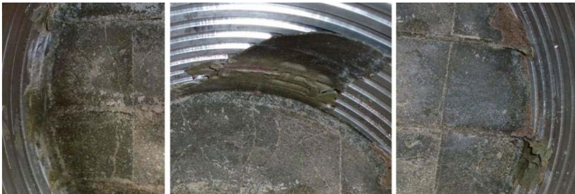
Figure 4-65. During the long time of 5 MPa water pressure the bentonite sealing had swelled into the voids between the concrete beams.
