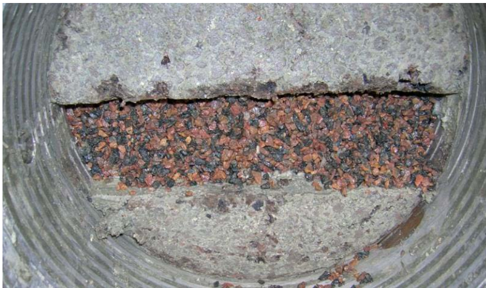
Figure 4-19. The Leca beams and the macadam filter seen from the backfill side. It seems as the backfill bentonite is successfully separated from the draining filter.
