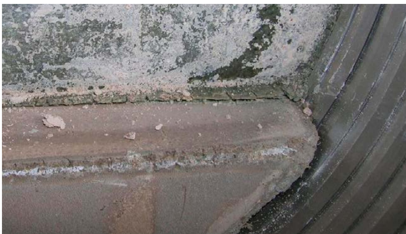
Figure 4-21. View of the bentonite sealing from the concrete plug side. The bentonite sealing has swelled into the void space between the beams.
