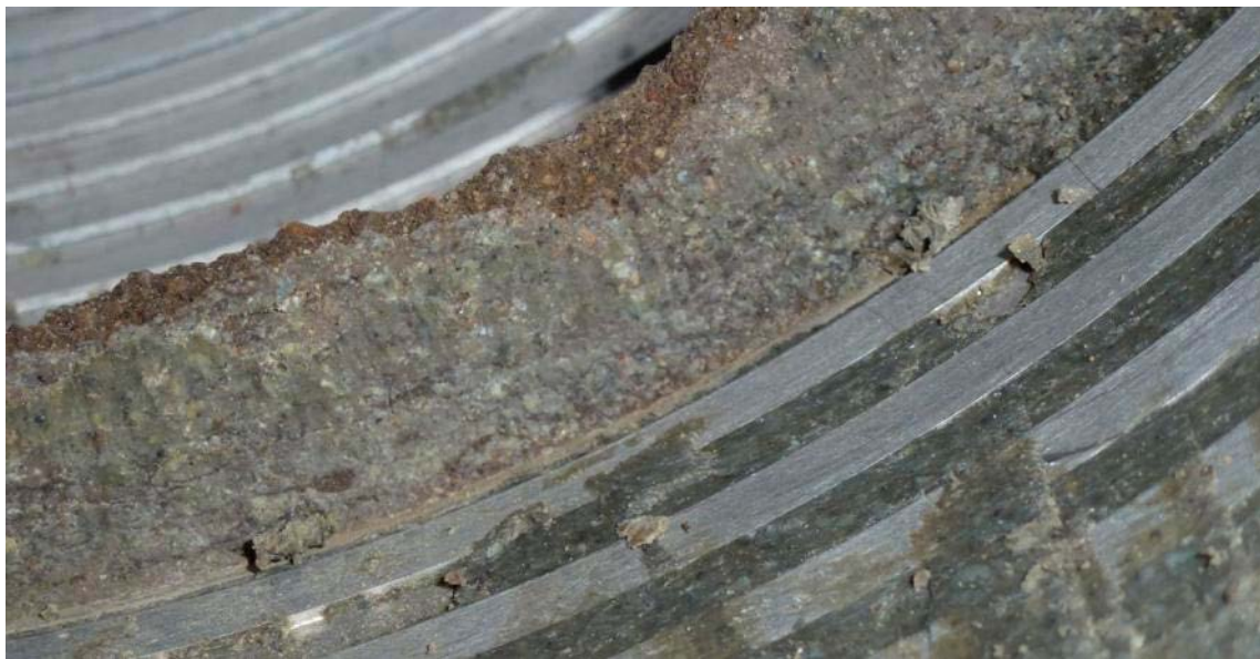
Figure 4-49. Example of the cast cement outermost part. The outer edge was visually inspected. No visible traces of piping or leakage were observed.
