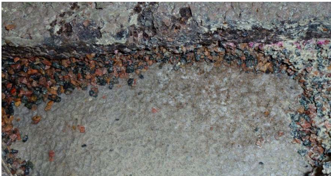
Figure 4-32. The Leca-beam and macadam filter at test dismantling. Bentonite has intruded into the macadam filter to the right (Window 1 side). It is likely that the bentonite intrusion occurred between the Leca-beams and the windows.
