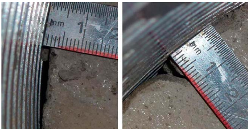
Figure 4-57. The void spaces between the concrete beams in Test 6. The voids are up to a few millimeters wide.
