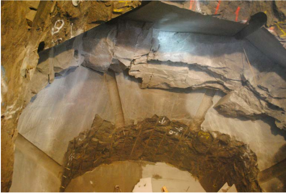
Figure 3-15. Detail photo of the remaining rock in the top and sides of the slot after blasting. This rock was removed by the use of a mechanical hammer.
