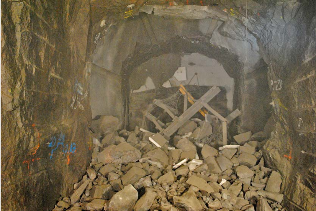
Figure 3-14. A view of the experiment tunnel TAS01 after blasting of the safety scaffold bearing structure and the free-sawn rock segments of the DOMPLU slot abutment.
