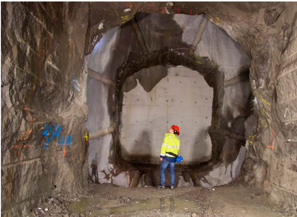
Figure 3-16. A view of the experiment tunnel TAS01 with the excavated slot abutment for the concrete dome.
