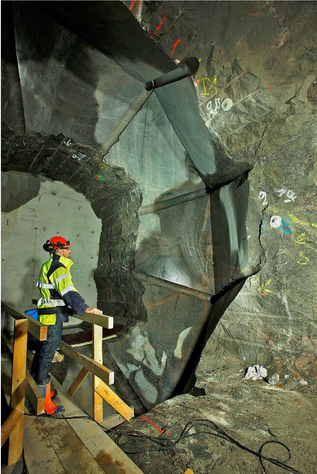
Figure 3-18. Right side of the excavated slot, to be used for casing of the concrete dome.
