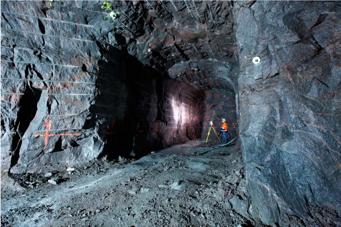
Figure 2-3. Photo of the completed test tunnel TAS01 where geodetic survey is ongoing.
