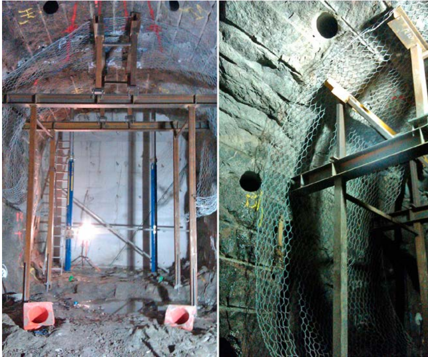
Figure 3-5. Photos from assembly of the safety scaffolding with a tunnel mesh to protect workers from falling stones.
