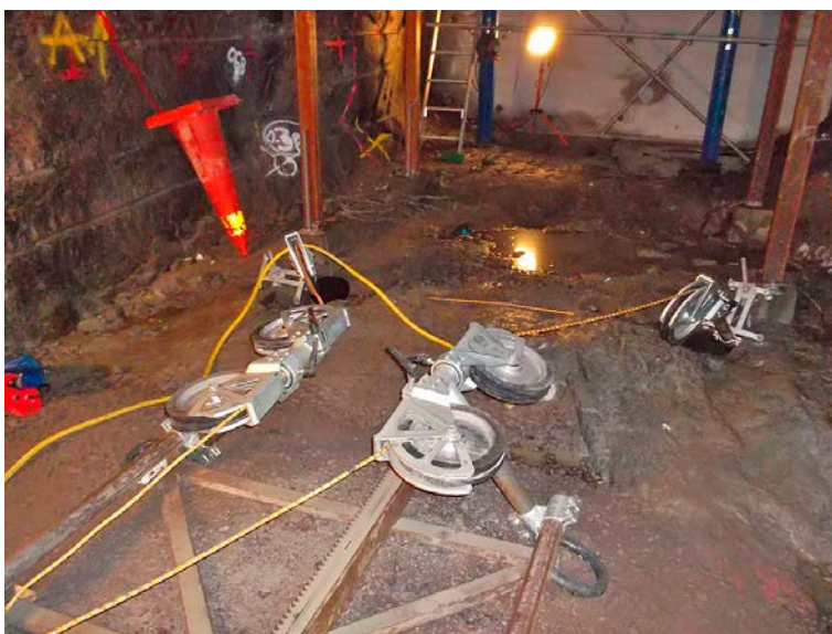
Figure 3-6. The guide pulleys inserted in the 250 mm bottom holes together with steering wheels for the wire connected to the wire saw machine.
