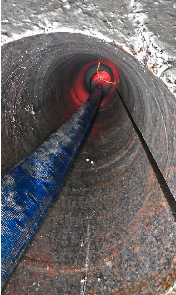
Figure 3-12. Detail photo of a \varnothing 250 mm borehole with one accomplished cut (on the right side) and with an installed pump used for drainage before preparing the next blind cut (on the left side).
