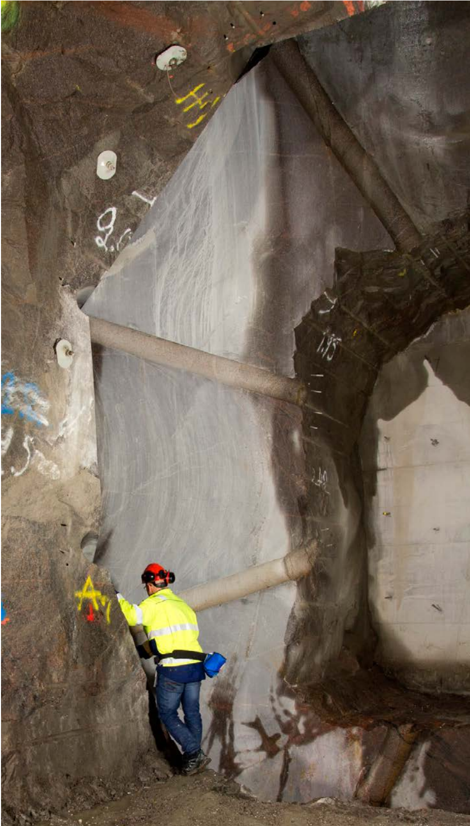
Figure 3-17. Left side of the excavated slot, to be used for casing of the concrete dome.
