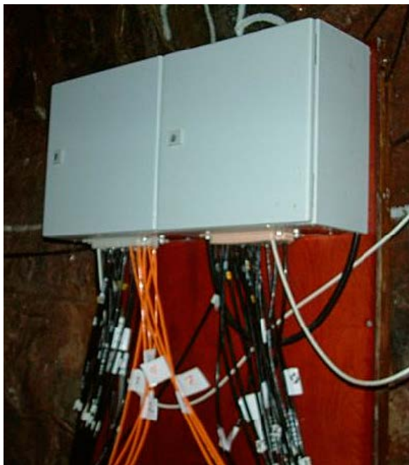
Figure 8-6. Boxes in the TASS tunnel with data logger communication system to the host computer. The logger has also local data storage.
