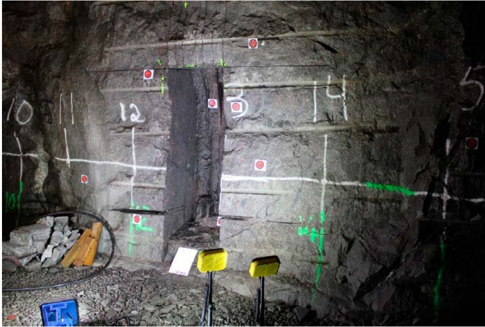
Figure 9-15. Photograph of a sawed slot at tunnel wall in TASN (Ittner and Bouvin 2015).
