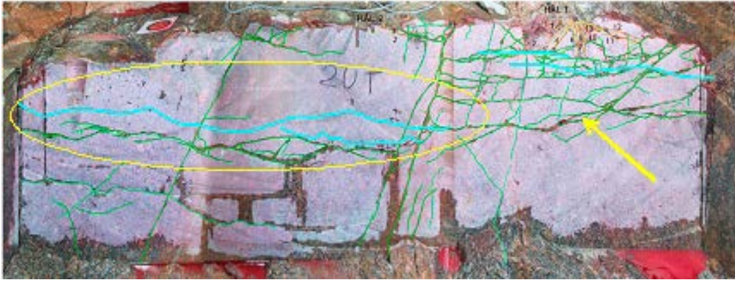
Figure ES-3. A photograph showing a sawed slot in the floor of TAS04 at tunnel length 34 m. The interpreted fractures from Ittner and Bouvin (2015) are marked with green (natural fractures) and yellow (excavation fractures). The light blue lines are GPR reflectors that intersect this section.
