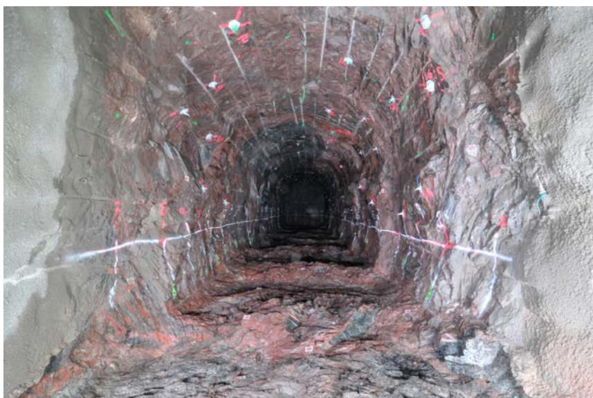
Figure 6-1. Foto showing the tunnel TAS04 taken from the tunnel mouth at approximately 4 m and looking towards the end of the tunnel at 37.5 m, with the floor cleaned and shotcrete at the tunnel mouth to approximately 7 m. The photograph is taken before the drilling of the 42 boreholes in the floor.
