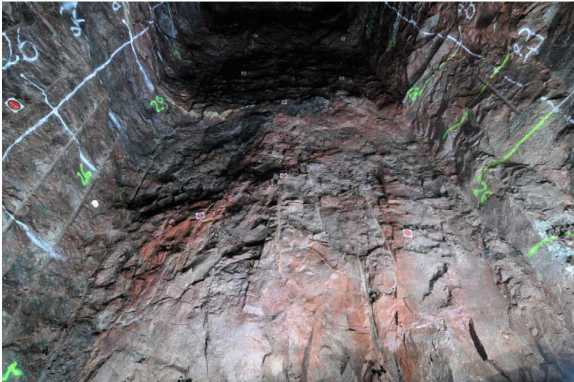
Figure 3-3. Example of the uneven tunnel floor after cleaning (looking into the tunnel). One of the depressions in the uneven floor was at the left side between chainage 26 and 28. This depression was probably caused by misalignment of the drilling. The photo also shows some of the steeply dipping NW trending fractures aligned nearly parallel to the tunnel axis (at the top in the photo).
