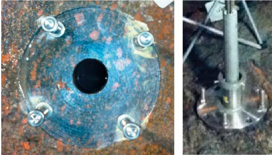
Figure 8-4. Flattened area around a borehole (at left); borehole extender in place and fastened to the flattened area (at right).
