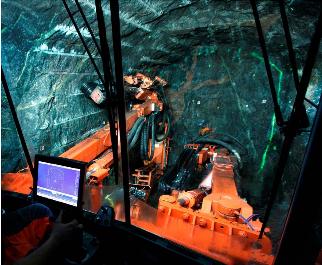
Figure 1-3. Drilling of a blast round with a two-boom jumbo. Note the contour holes and the step between two rounds caused by the look-out angle.
