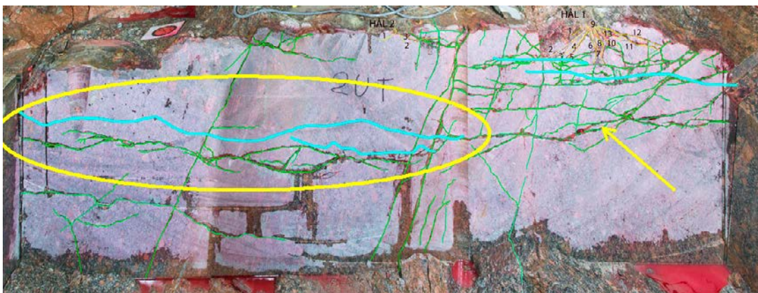
Figure 9-16. A photograph showing a sawed slot in the floor of TAS04 at tunnel length 34 m. The interpreted fractures from Ittner and Bouvin (2015) are marked with green (natural fractures) and yellow (excavation fractures). The light blue lines are reflectors that intersect this section.
