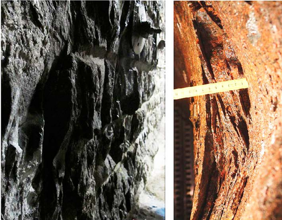
Figure 1-1. Left: A smoothly blasted tunnel wall. The perimeter holes for blasting are seen as lighter lines. The irregular surface of the wall is primarily caused by the vertical blast-induced cracks. Right: stress-induced spalling from a 1.8 m diam. Borehole (looking up the hole). The spalled zone is approximately 10 cm deep.
