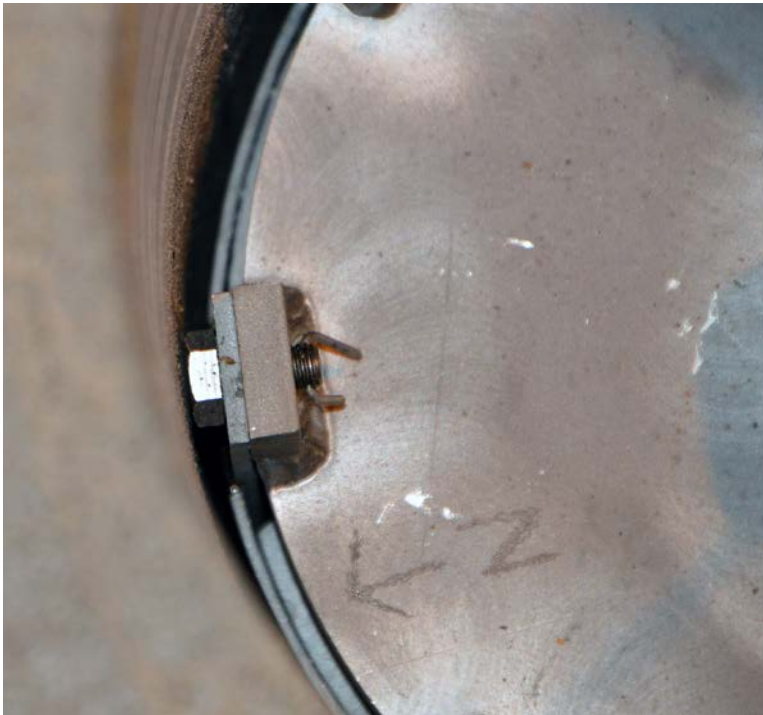
Figure 7-1. The head of the bolt holding the lid of the titanium cage will obstruct the removal of sand and bentonite from the slit between the bentonite package and the bedrock in the deposition hole.
