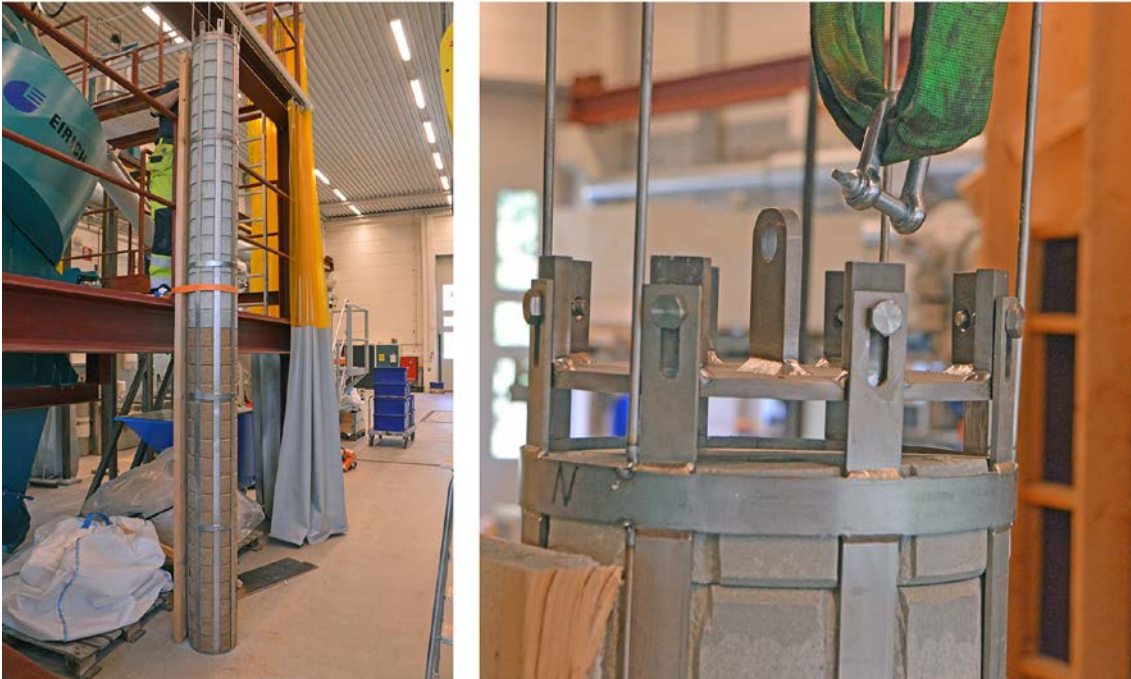
Figure 6-5. The titanium cage was raised towards the steel construction and the bentonite blocks emplaced from the top. After that all the blocks had been emplaced the lid with the lifting eye was mounted to the cage with 8 bolts.
