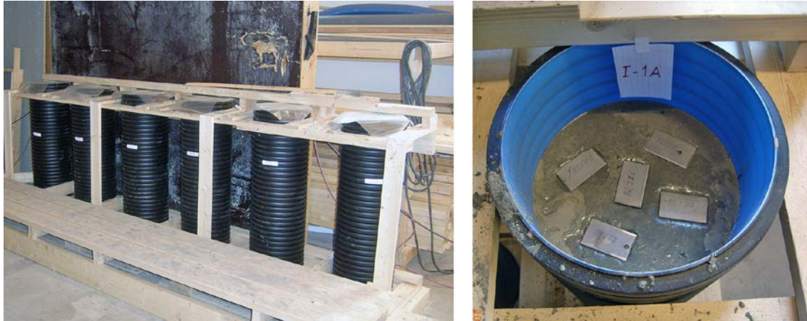
Figure 5-2. The Sewage pipes used for casting of the concrete cylinders in Concrete and Clay phase 1 and 2 (left image) and the interior of the mould during casting of concrete cylinders containing specimens of stainless steel (right image).
