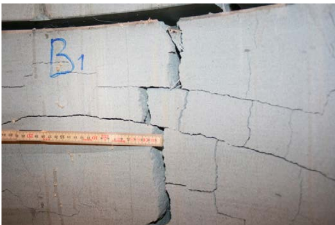
Figure 4-9. Cracks observed from the inside of the ring shaped blocks.
