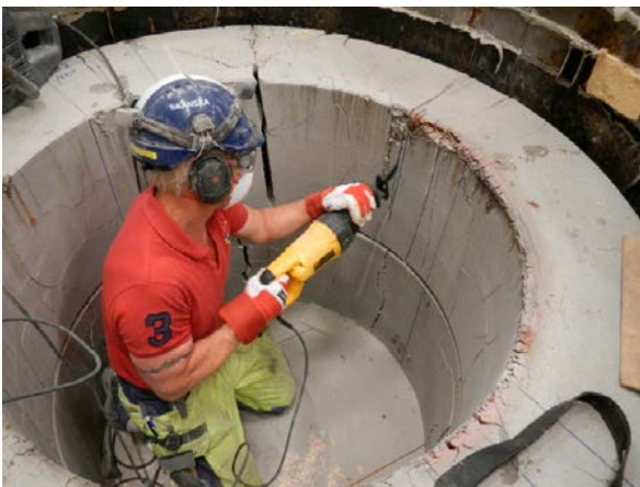
Figure 4-11. A large piece of bentonite cut out from the upper block with an alligator saw.
