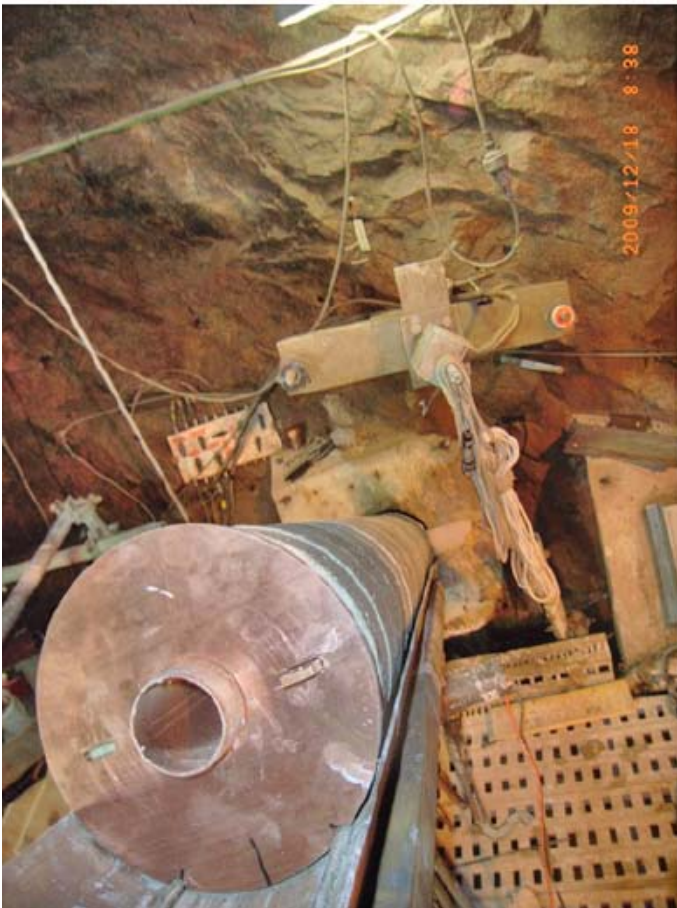
Figure 3-1. Placement of clay blocks. Upper: Funnel for letting the blocks slide down. Lower: Block column with copper plate and fixed central tube passing through.
