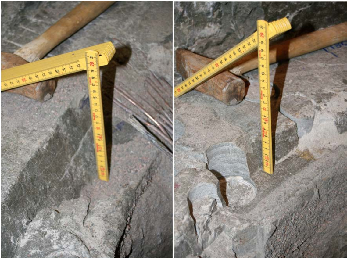
Figure 2-10. Shelves of top surface of Ring 12 indicating shearing. Left: in 350° direction inclination approximately 65° in relation to the horizontal plane; right: in 200° direction inclination approximately 72° in relation to the horizontal plane.
