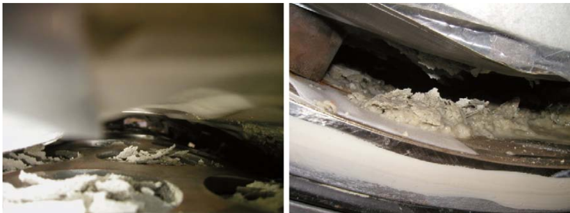
Flaking of bentonite through perforations.
