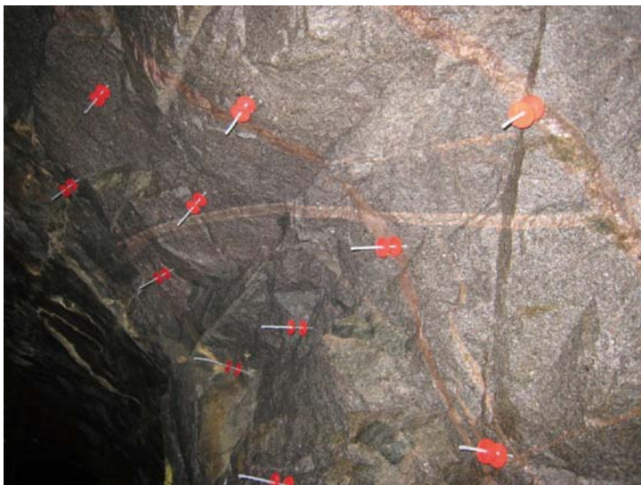
Figure 4-8. Threaded rods with plastic washers marking the intended shotcrete thickness, placed at approximately 0.5 m distance.
