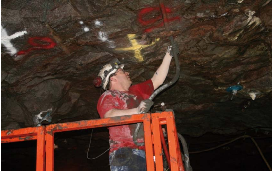
Figure 3-8. The boreholes were filled from the end of the hole retreating towards the collar in order to minimize the amount of air trapped in the hole.
