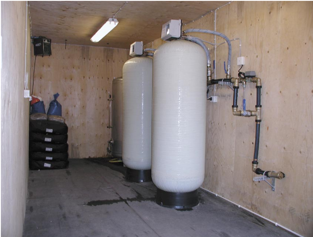
Figure 3-7. The active carbon filter plant used for reduction of total organic content (TOC) in the flushing water.
