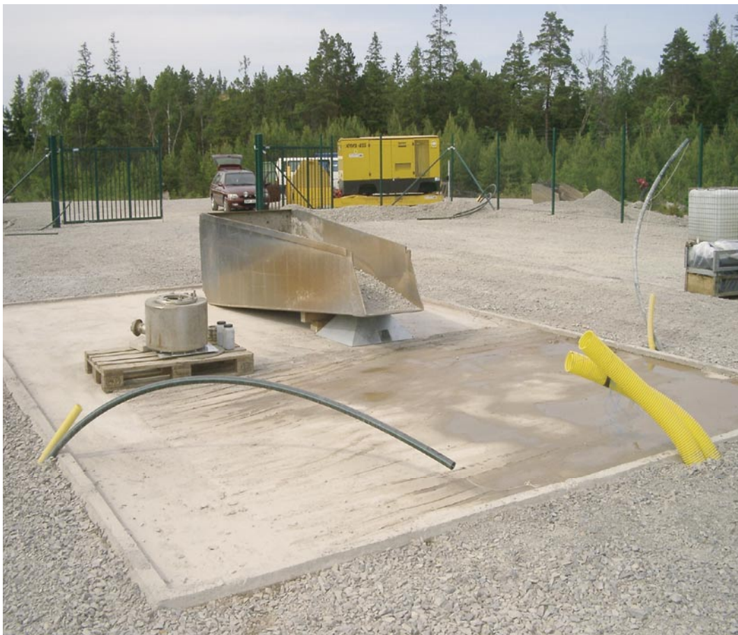
Figure 1-4. The ground surface was levelled off and covered with coarse gravel, and a 7 x 5 m cement slab was cast around the planned borehole position.
