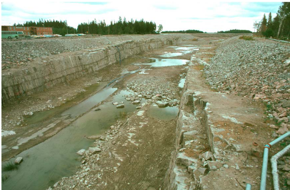
Figure 3-10. Picture from the construction of the 13 m deep and more than one kilometre long canal between the Baltic Sea and the nuclear power reactors in Forsmark. Horizontal fractures/sheet joints are encountered along the entire excavation. The sheet joints follow the undulations of the bedrock surface implying that many of them do not outcrop, but stay below the bedrock surface as this dips under the Baltic Sea. There are several “horizons” of extensive sheet joints on top of each other according to the hydraulic interference tests /Follin 2008, Figure 5-14/.
