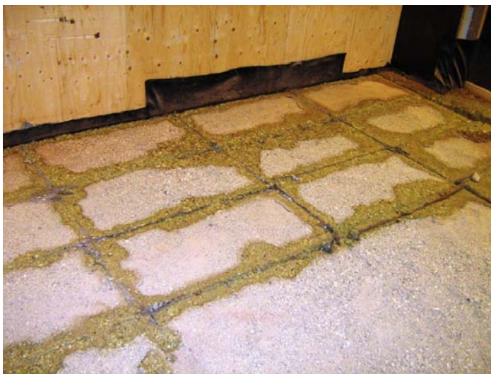
Figure 5-15. After removal of the blocks large dry areas were seen.
