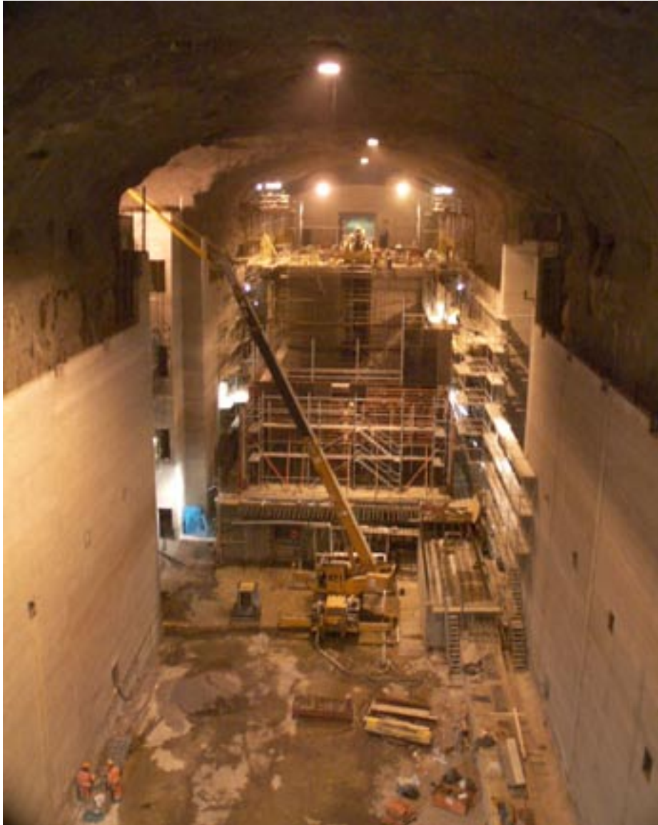
Figure 3-3. Picture from construction of the CLAB-2 cavern, where monitoring data were used to adapt the excavation work to the rock conditions and to check compliance with requirements.
