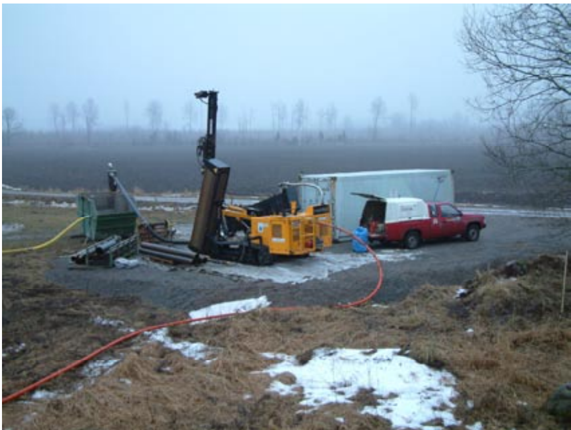
Figure 3-1. The Nemek 407 percussion drilling machine engaged for drilling the three percussion boreholes in solid rock at drillsite DS3. Water and drilling debris is discharged to the container. Photo Alf Sevastik.
