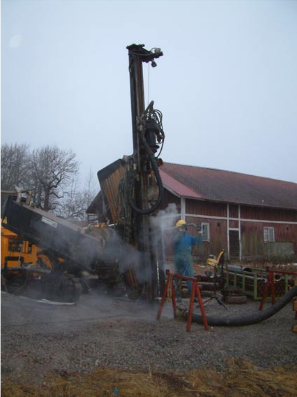
Figure 4-1. A high temperature steam cleaner is used for cleaning the drill pipes at level two according to SKB MD 600.004, Version 1.0, before start of Ejector-NO-X drilling. Photo Alf Sevastik.
