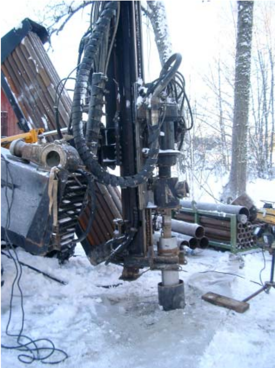
Figure 3-2. The Nemek 407 percussion drill machine with a 168/160 mm temporary steel casing simultaneously driven through the overburden and approximately one metre into the bedrock while drilling at DS3. Photo Alf Sevastik.
