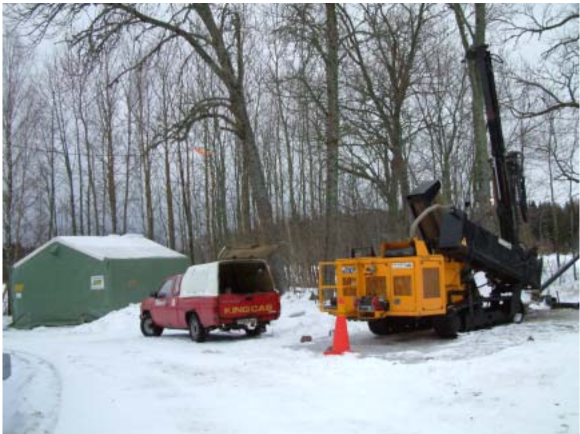
Figure 3-1. The Nemek 407 percussion drill machine engaged for drilling the monitoring wells in unconsolidated soil layers. Note the fluidproof cover beneath the drill rig used for protection of the ground in case of unintentional oil spillage. Photo Alf Sevastik.
