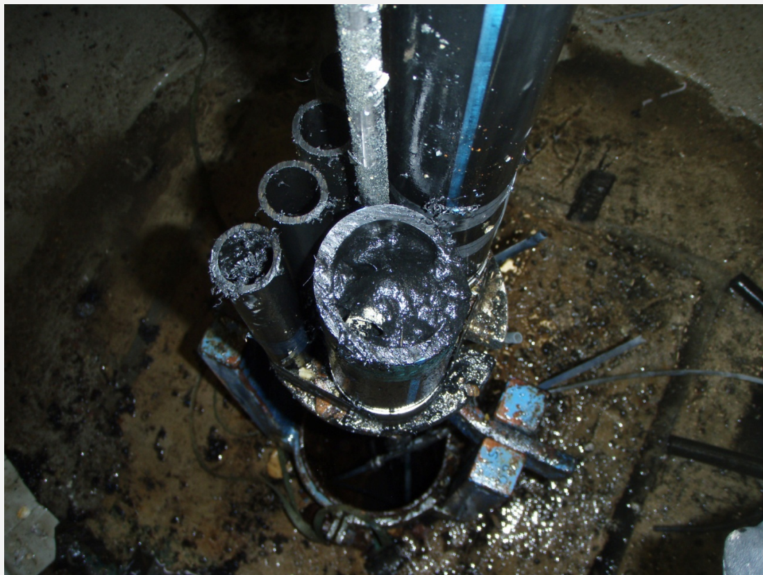
Black precipitate and a strong smell of hydrogen sulphide gas in the standpipes of borehole KAS03. The borehole equipment (iron bars, plastic tubing and rubber packers) was installed more than 20 years ago for groundwater and pressure monitoring purposes.
