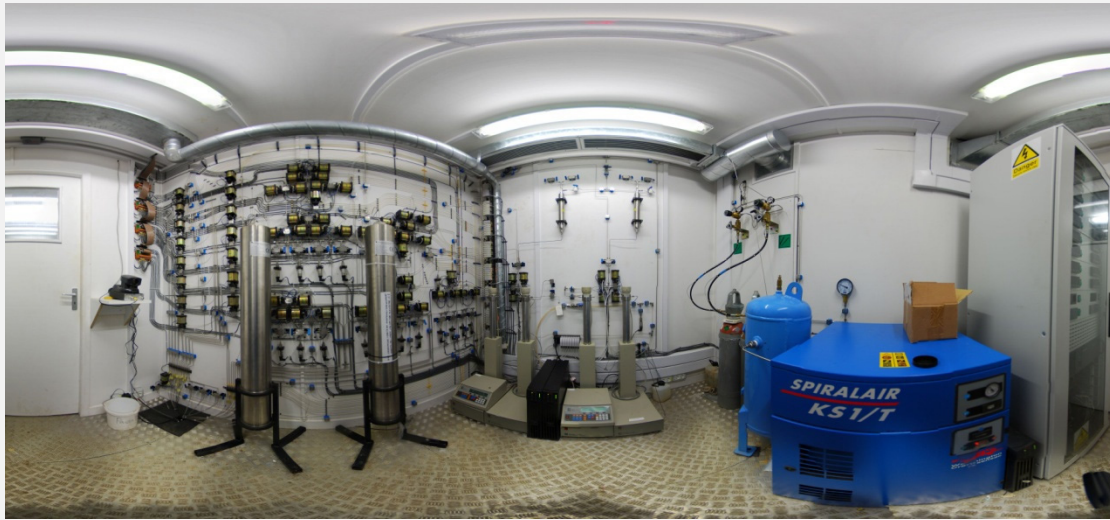
Panorama of the laboratory of the Large Scale Gas Injection Test (Lasgit) at -420 m level in Äspö HRL.
