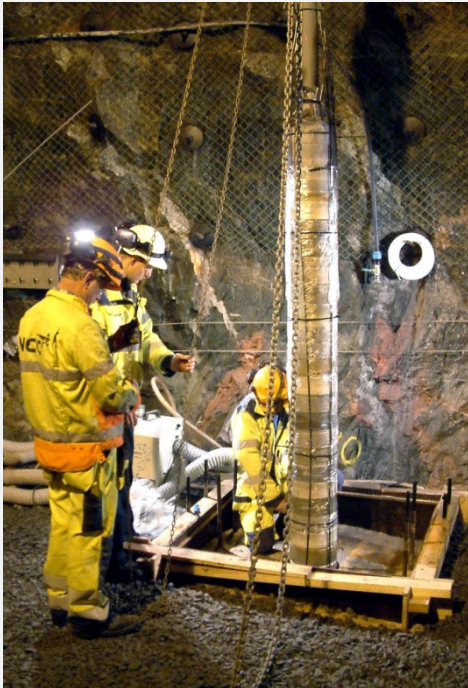
Installation of one of the three test parcels. The photo illustrates the mixing of different compacted buffer blocks.
