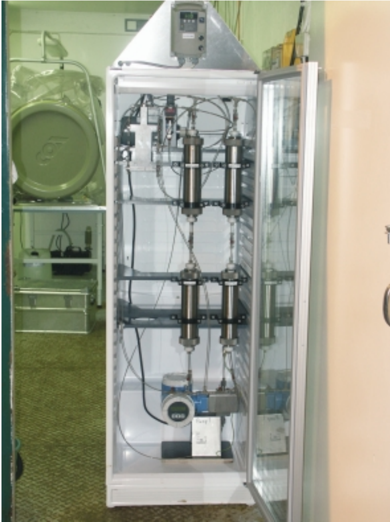
Figure 2-21. One of the circulating systems at the MICROBE 450-m site, built in a refrigerator equipped with a fan that ensures even temperature distribution. Four flow cells offers 125 cm 2 surface each for attachment and growth of microbes. The cells have a stainless steel outer shell, but expose only Polyvinylidene fluoride plastic inside (PVDF) to the flowing groundwater. A pump on top inside the cabinet, with a pump rate control on the top outside, circulates groundwater from the borehole via the flow cells and back into the aquifer. A flow meter at the bottom registers flow rate and pumped volume over time.
