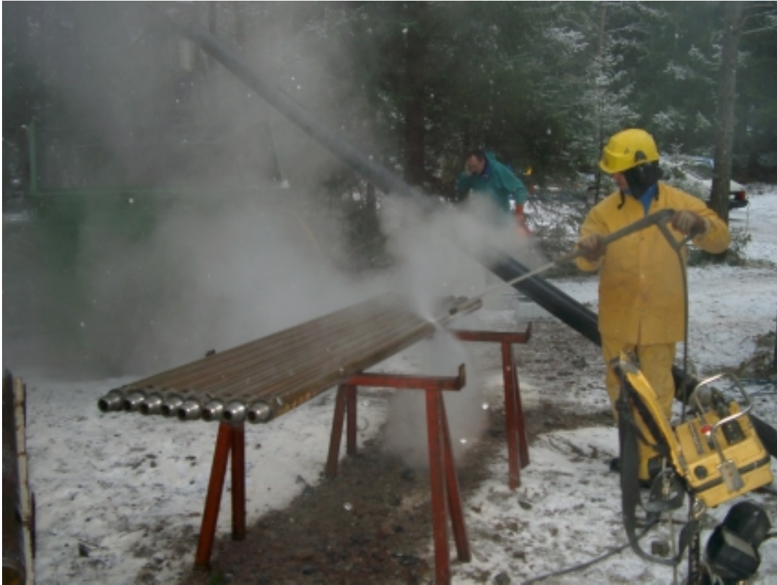
Figure 4-1. A high temperature steam cleaner is used for cleaning the drill pipes at level two according to SKB MD 600.004, Version 1.0, before start of Ejector-NO-X drilling. Photo Alf Sevastik.
