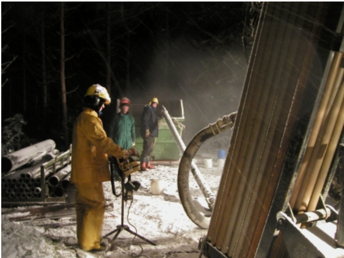
Figure 3-1. The Nemek 407 percussion drilling machine engaged for drilling the two percussion boreholes in solid rock at drillsite DS2. Water and drilling debris is blown to the container. Photo Niclas Karlsson.
