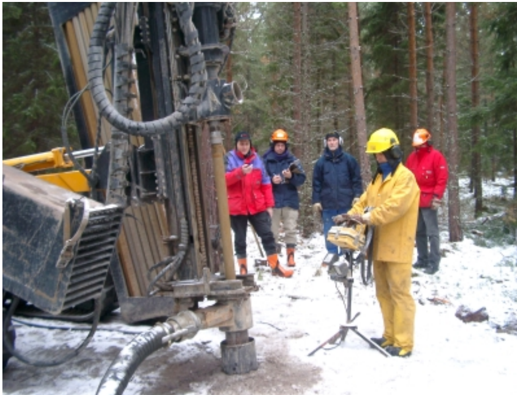
Figure 3-2. The Nemek 407 percussion drill machine with a 168/160 mm temporary steel casing simultaneously driven through the overburden and approximately one metre into the bedrock while drilling at DS2. Photo Alf Sevastik.
