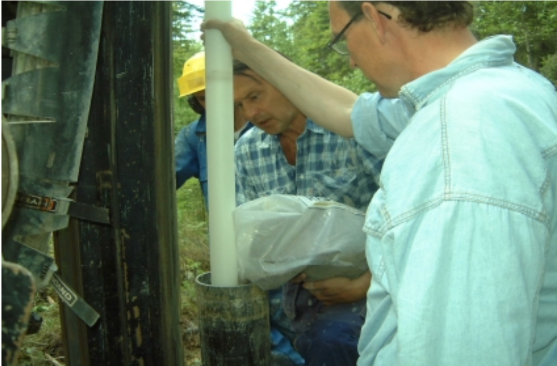
Figure 4-1. Installation of the HDPE well screen, riser pipes, sand filter and bentonite sealings in a groundwater monitoring well inside a temporary steel casing. The snapshot illustrates filling with bentonite pellets. Photo Göran Nilsson.
