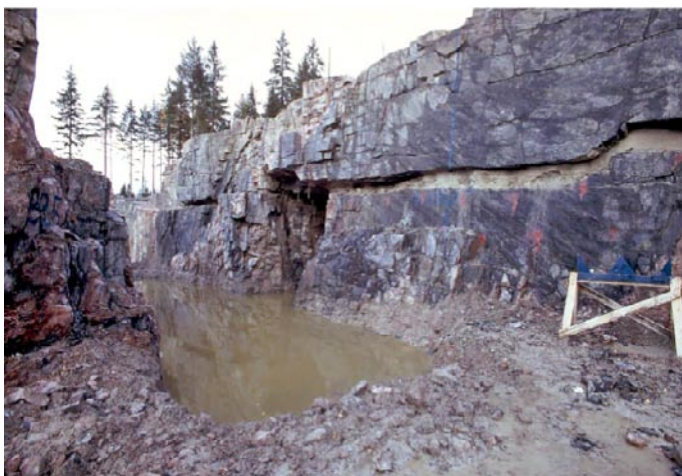
Figure 1-8. Shallow fractures sub-parallel to the ground surface in the excavation for unit 3 of the Forsmark power plant /Carlsson 1979/. The fractures may have been created by extensional strains caused by large horizontal loads (sheeting joints). They may also have been formed or opened up further by high pore pressures (hydraulic jacking).
