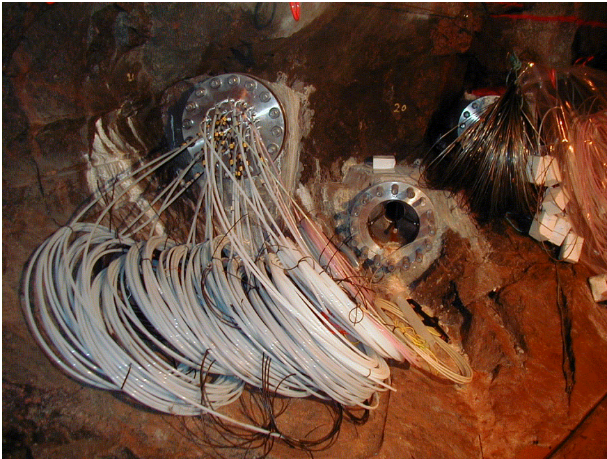
Figure 3-1 Installed lead-throughs with cables and instruments in the Prototype tunnel ready to be placed in the bentonite blocks in deposition hole # 3. The empty lead-through is for the electrical cables to the heaters and the fibre optical cables.
