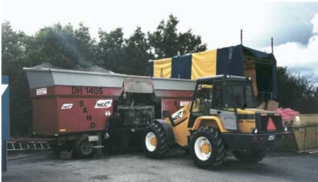
Figure 9-1. Mobile station for producing larger quantities of thoroughly mixed bentonite/ballast material (100 m 3 per day). NCC was the construction company.
