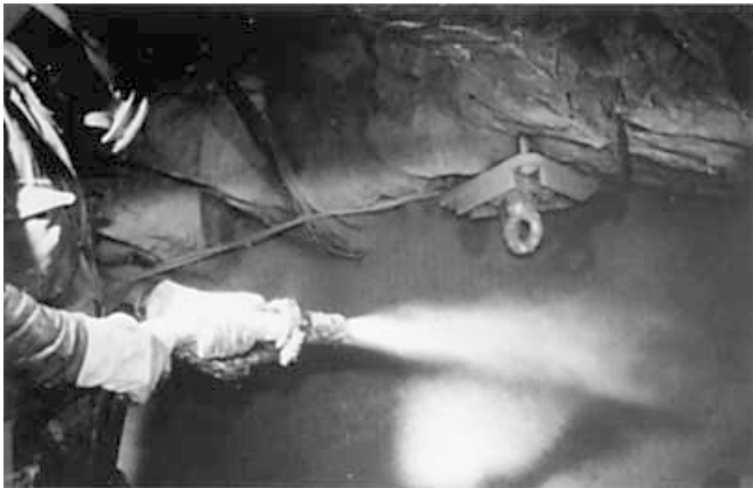
Figure 9-12. Blowing of 20/80 mixture near the roof of the drift /1/.
