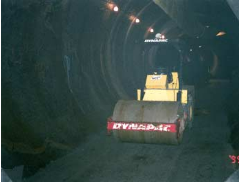
Figure 9-6. Compaction by use of a 4.7 t vibratory roller in a TBM tunnel.
