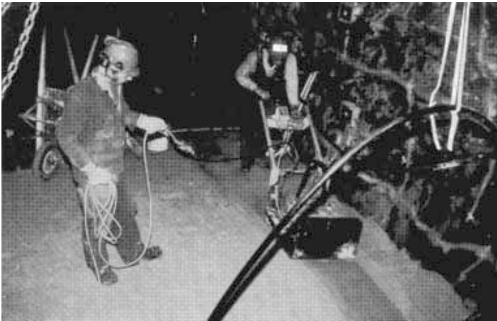
Figure 9-5. Compaction of 10/90 bentonite/ballast mixtures. Upper: 400 kg vibratory plate /1/. Lower: 4.7 t vibratory roller.
