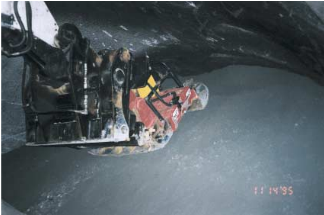
Figure 9-8. Example of “sideways” backfilling and compaction. The lower picture shows a 700 kg vibrator plate mounted on a tractor for compaction of inclined backfill layers. The plate was electrically powered and could be tilted, turned and pushed to produce 30–40° inclination of the slope.
