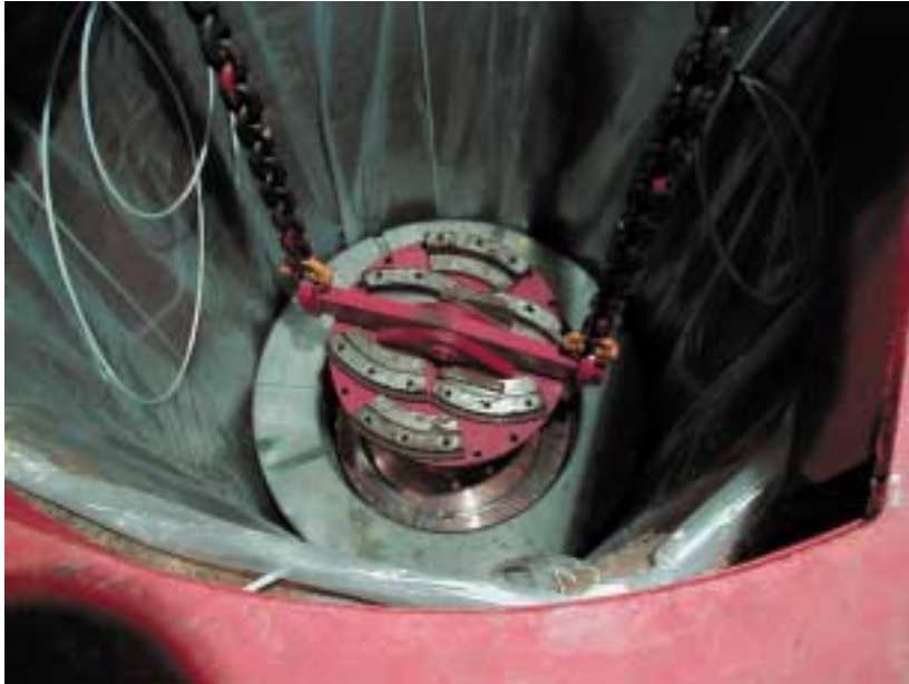
Figure 4-2. The canister is placed in the deposition hole. The gripping device has been made free from the lid and is being hoisted. The plastic covering the walls is installed for protection of the bentonite, since there is a long time between deposition of the bentonite blocks and backfilling of the tunnel.
