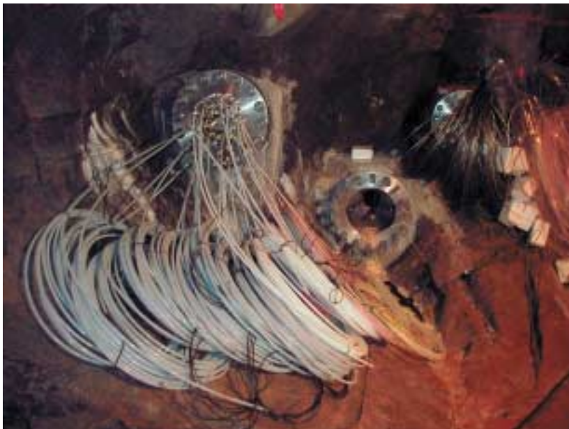
Figure 4-3. Installed led-throughs with cables and instruments in the Prototype Repository tunnel ready to be placed in the bentonite blocks in deposition hole 3.
