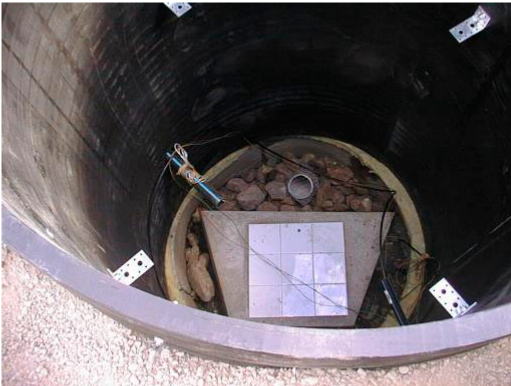
Figure 3-1. A digged ditch down to the rock surface with a concrete construction where the seismometers will be placed.
