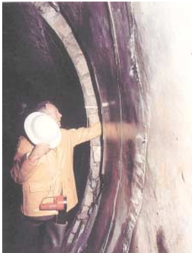
Figure 3-6. Pavoncelli tunnel. Rupture of lining at transition from Varicoloured clays to Pliocene blue clays of the Ofanto Basin. Photo from chainage 8910 /Cotecchia, 1986/.
