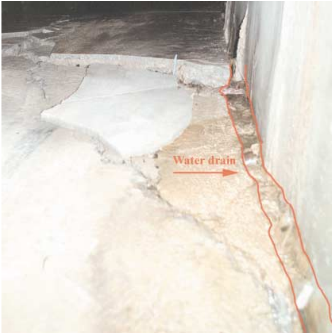
Figure 3-20. The picture shows the concrete floor that was broken due to the Chi-Chi earthquake. The effects of shockwaves are slightly visible in the tunnel wall as the width of the water drain varies in width. One of the guides, Mr T T Wang, was member of the engineering team during construction and confirmed the existence of the shockwaves not being construction flaws. Photo: G Bäckblom.
