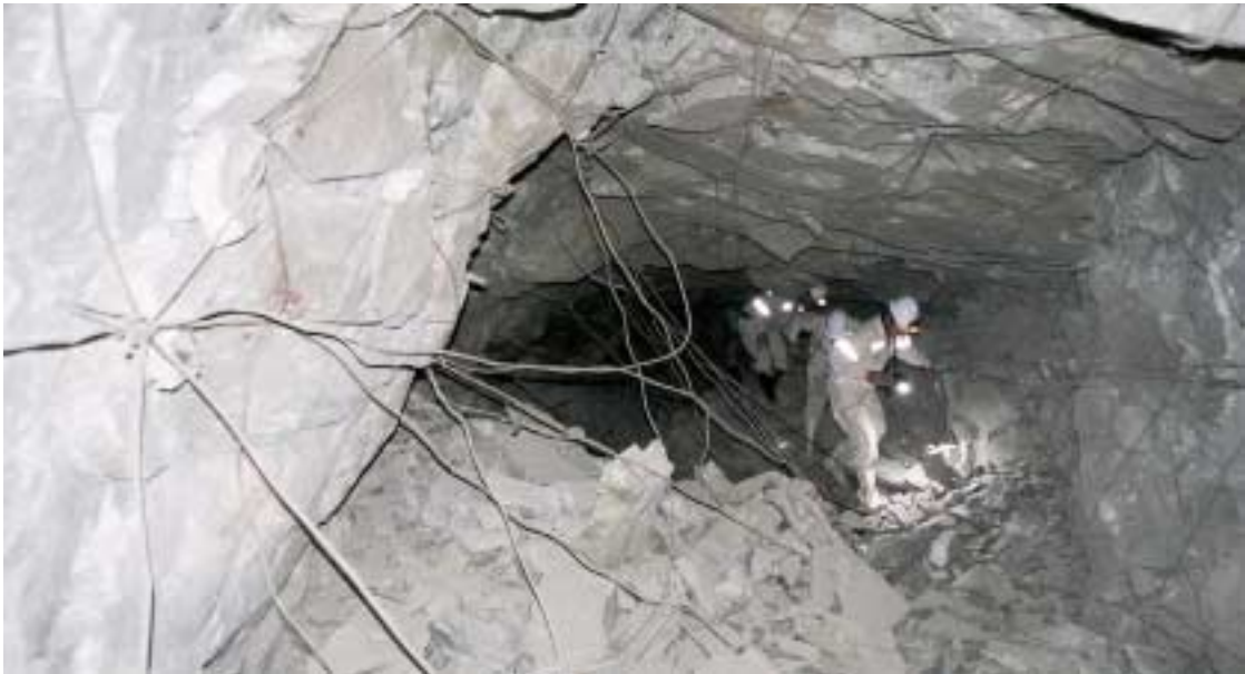
Figure 3-18. Examples on shaking damage in the A.R.M Shaft # 5. Drift at the Level 64 (2150 m below surface). The drift is partially collapsed. Photo: G Bäckblom.
