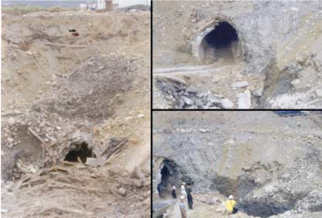
Figure 1-8. The Chi-Chi earthquake in Taiwan 21 September 1999 displaced the Shib-Gang Dam water conveyance tunnel intersecting the Chelungpu fault that ruptured the surface for ~100 km. This tunnel was sheared off 4 m vertically and 3 m horizontally. Damage in the tunnel lining was limited to within a few meters of the reactivated fault /Wang et al, 2001/. The Shib-Gang Dam water conveyance tunnel is around 10 m below surface and excavated through unconsolidated alluvium. The tunnel was excavated by a ripper and lined with concrete. Courtesy: Mr T T Wang.
