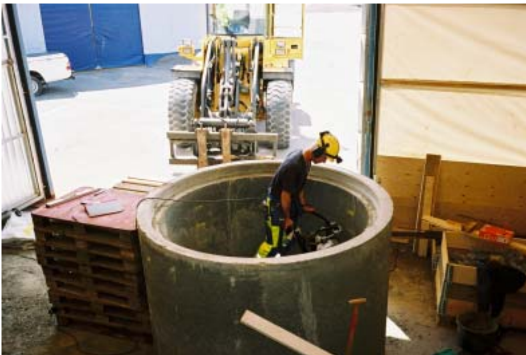
Figure 3-1. Compaction in the concrete ring.
