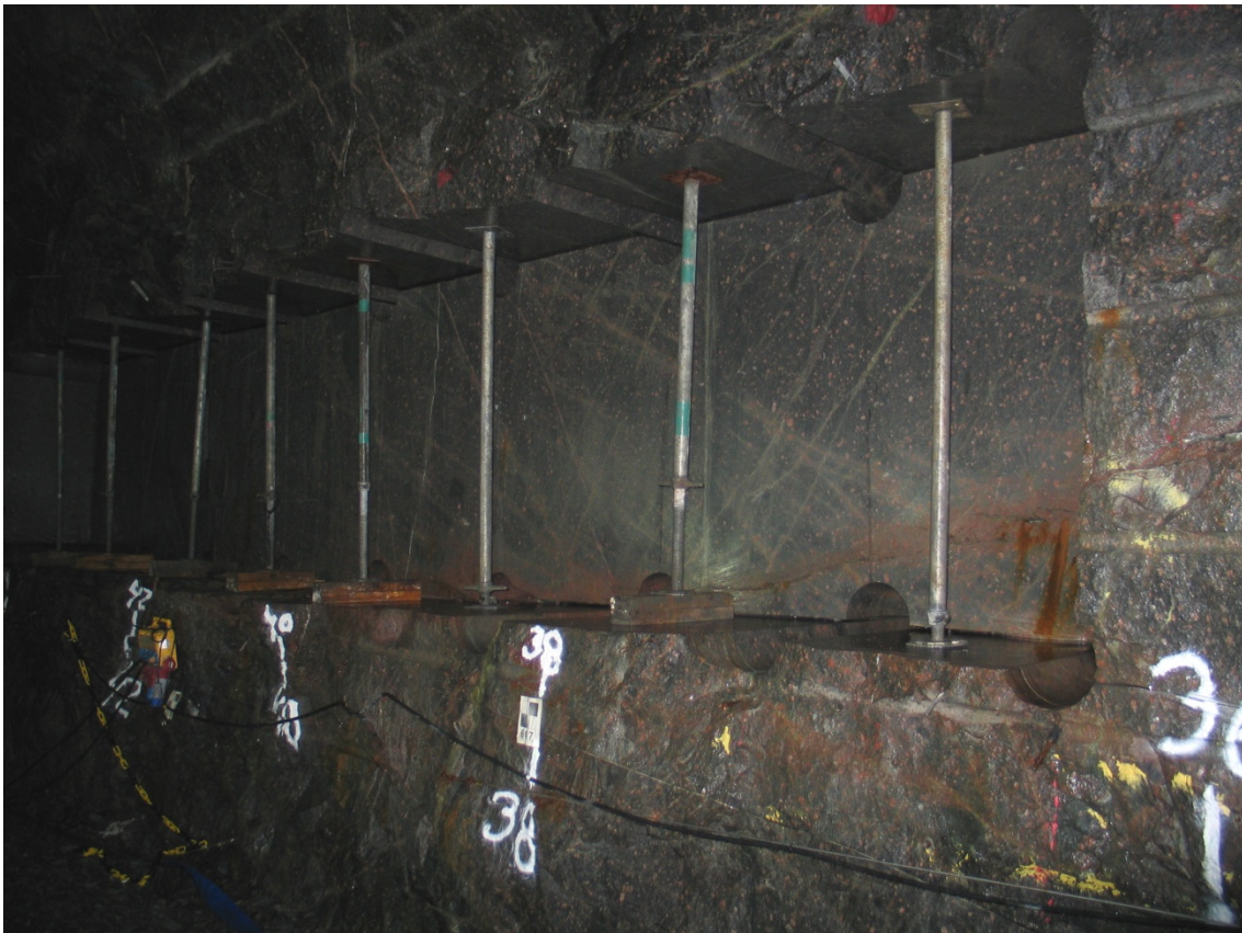
Figure 2-1. TASS-tunnel, section 36-42 m (approximately). The Excavation Disturbed Zone (EDZ)-slot on the right wall which was mapped in detail during the previous four-month period of 2009.
