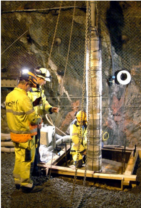
Installation of one of the three parcels illustrating the mixing of the different compacted buffer discs.
