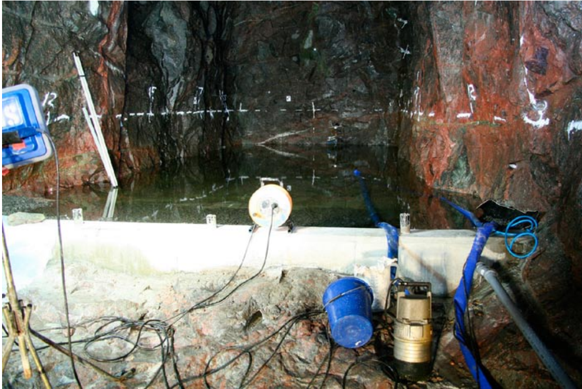
Figure 4-26. A lot of effort is given to the measurement of the inflow to the tunnel. Here, a measuring dam, a so called weir. The dam is filled with water in order to get an outflow from the dam that is stable. Photo: Magnus Kronberg.
