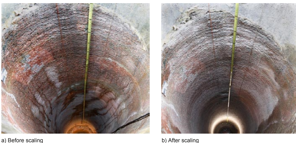
Figure 2-5. Photographs of the south-west-side of heater hole KQ0048G05, the dryer hole in the third test before a) and after b) scaling of the borehole wall.
