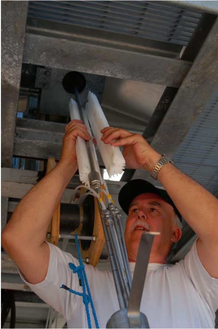
Figure 4-9. Installation of equipment for groundwater level monitoring in a core drilled borehole.
