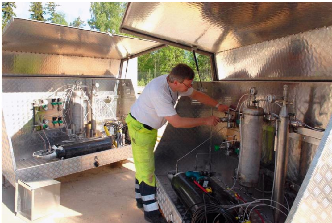
Figure 4-11. Interior of two housings used as borehole collar shelters after installation of groundwater level monitoring equipment in percussion drilled boreholes.
