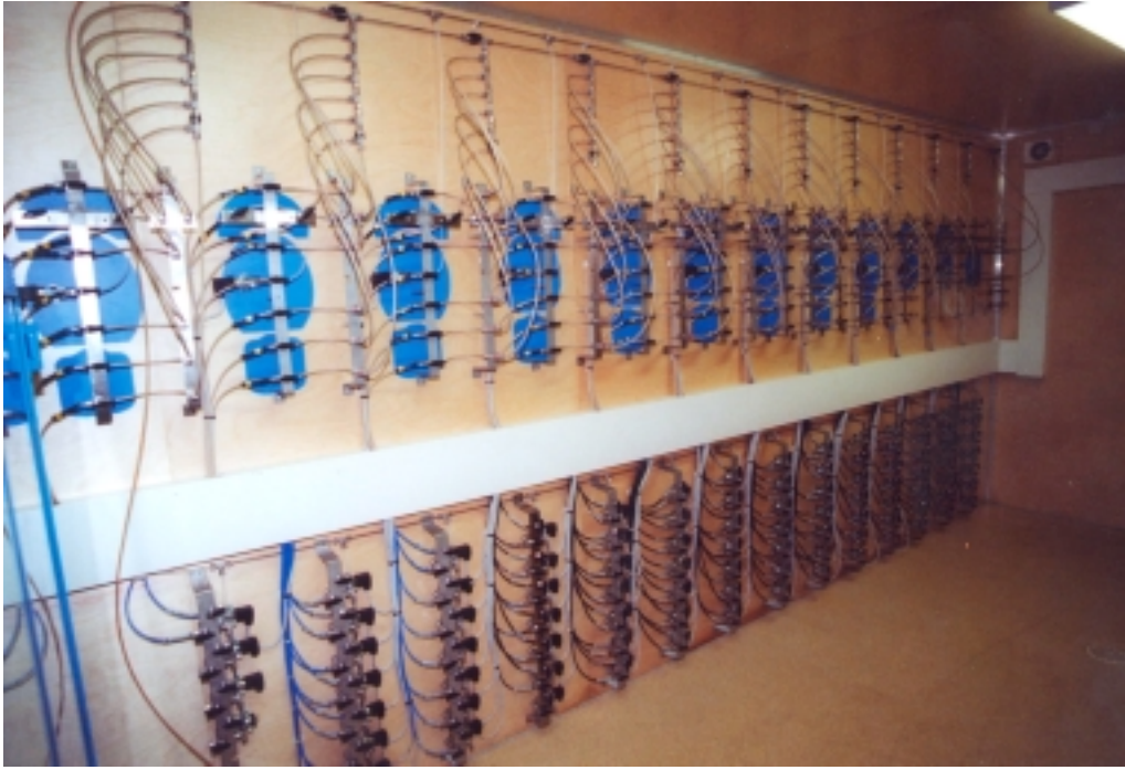
Figure 11-34. Photo of control panel for the permeable mats (upper system) and the system for connecting the Druck transducers
