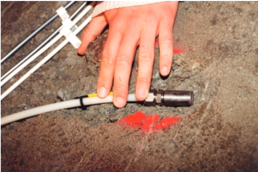
Figure 11-24. Photo of a Psychrometer installed in the backfill
