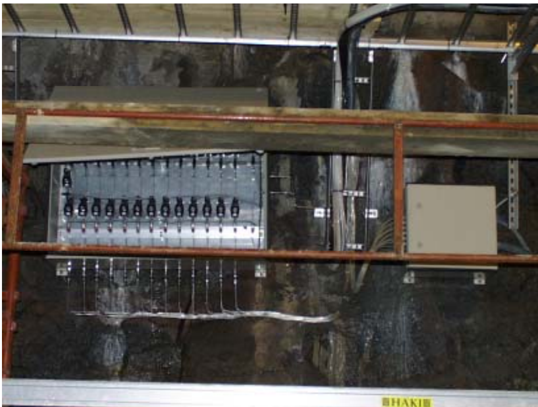
Figure 7: Valves box (left) and junction box at Demonstration drift.
