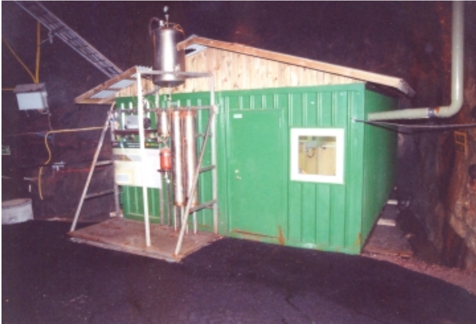
Figure 11-27. Photo of the data acquisition house
