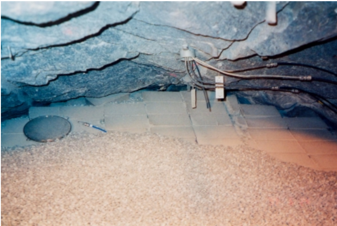
Figure 7-20. Filling the remaining space at the roof with 20/80 blocks and bentonite pellets.
