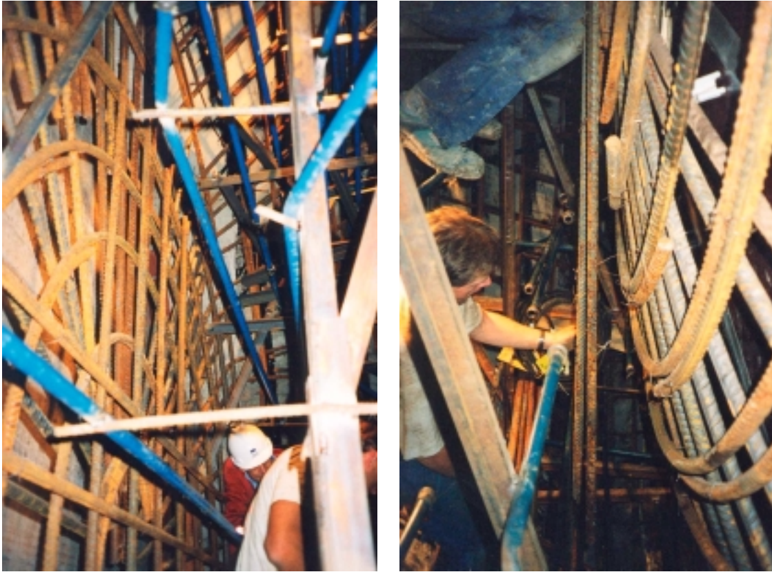
Figure 11-16. Reinforcement at the retaining wall (left) and parabolic outer surface (right). Photographs were taken during installation of cooling pipes, i.e. after completion of the reinforcement work.
