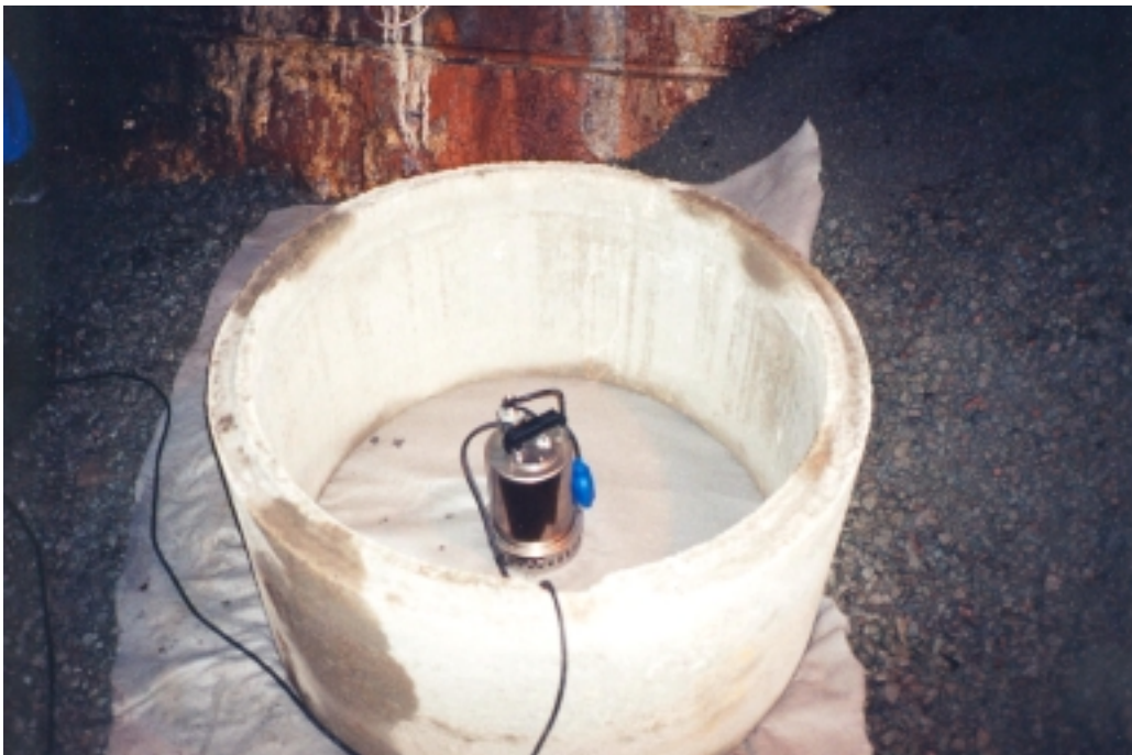
Figure 5-11. Sump with pump.
