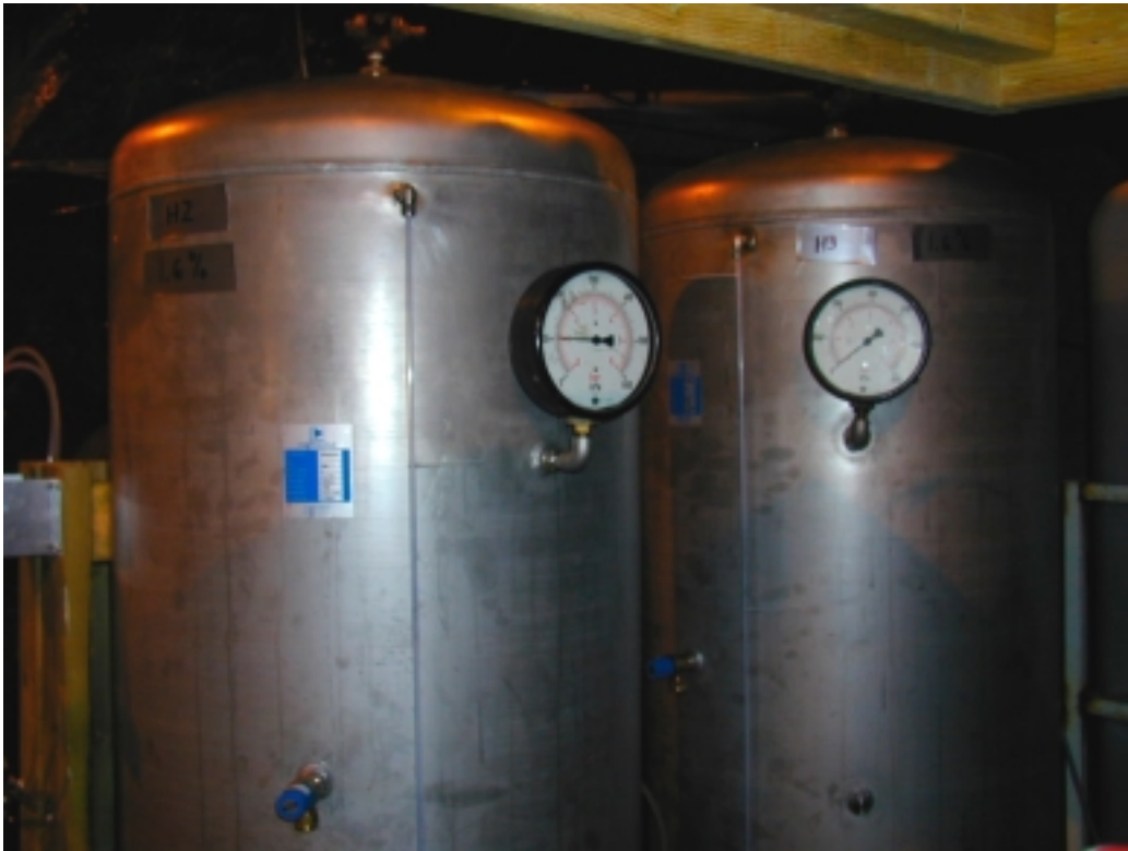
Figure 11-31. The pressure vessels with the 600 kPa manometers.
