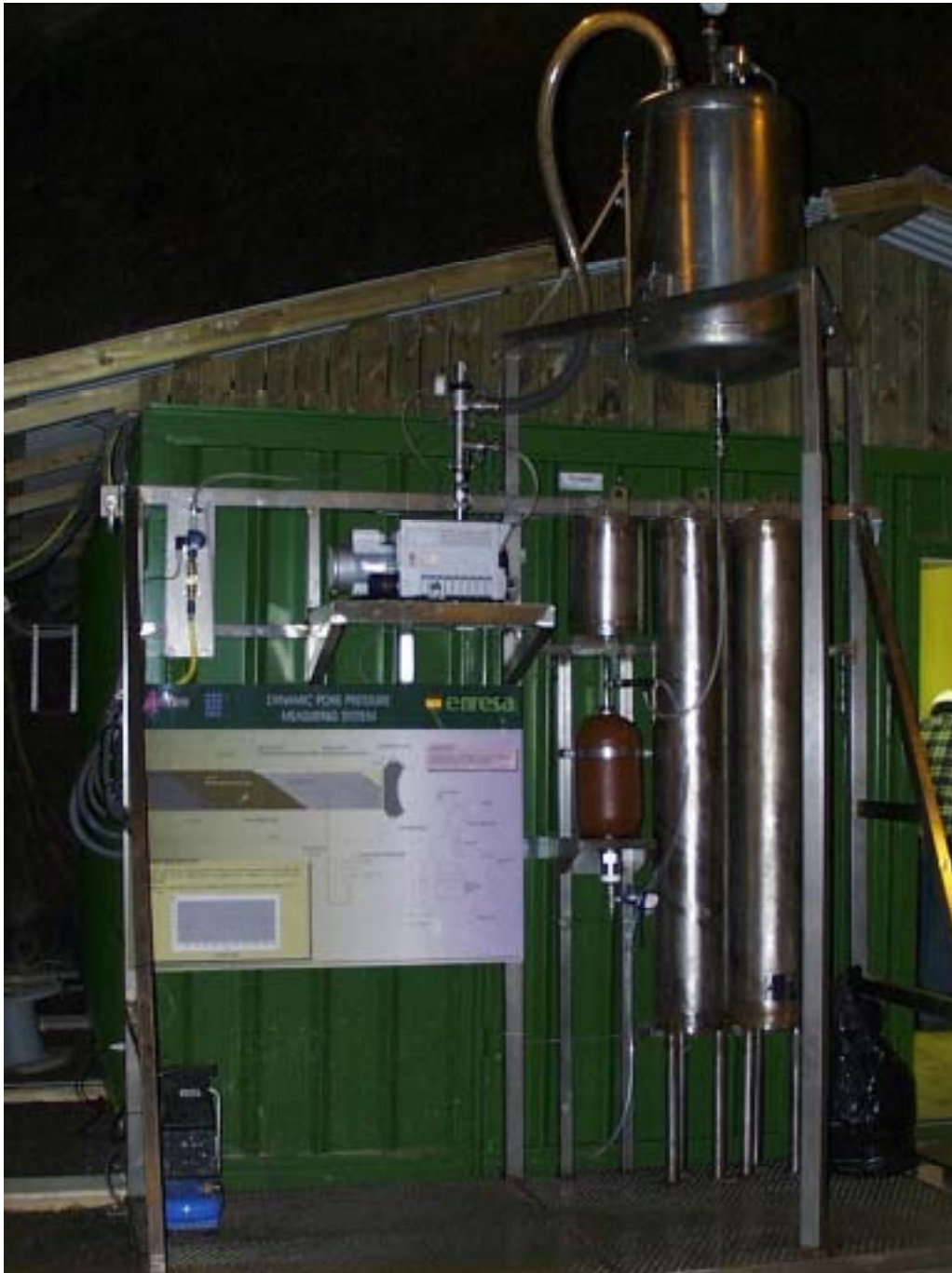
Figure 8: Measuring and control system (metallic structure outside control room).
