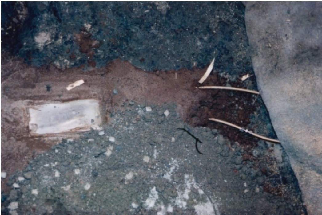
Figure 5-5. Pressure cell mounted in the floor.
