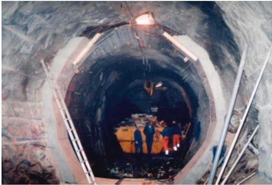
Figure 12-8. Abutment viewed from inside the ZEDEX tunnel prior to starting the backfilling operation
