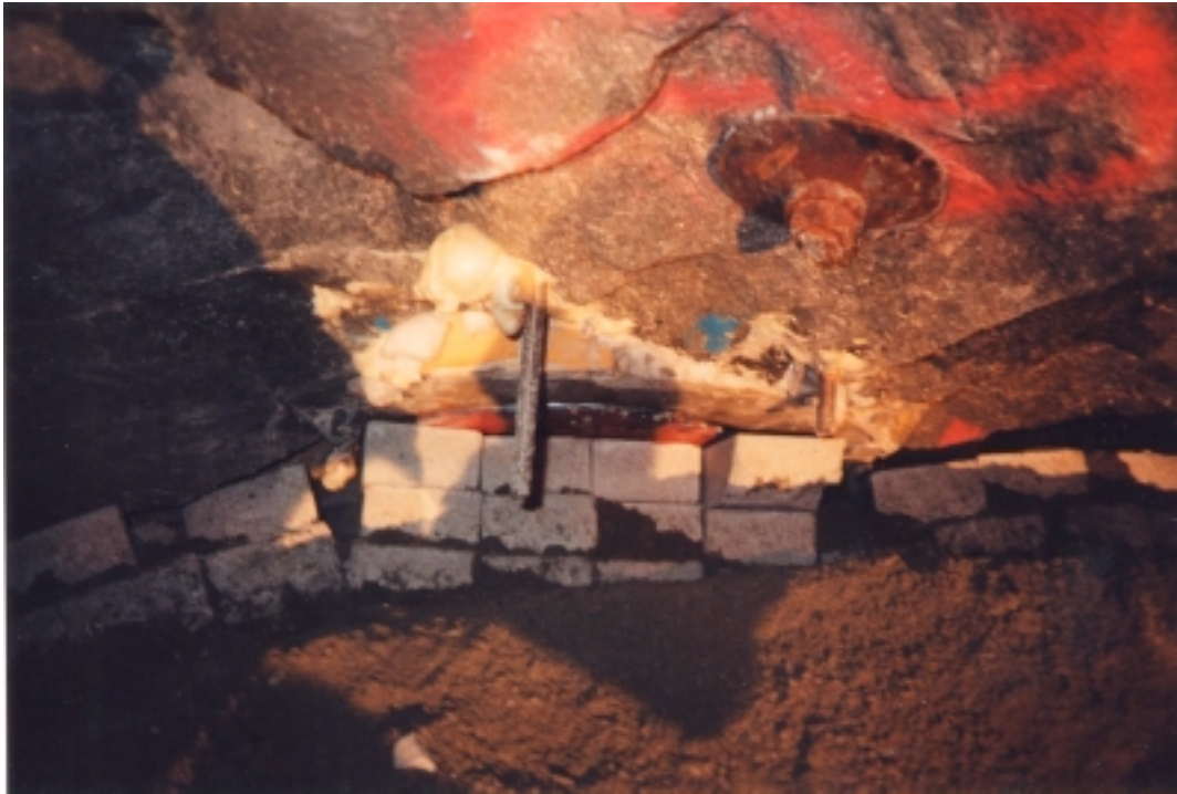
Figure 5-4. Pressure cylinder mounted in the roof above the bentonite blocks.
