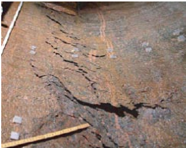
Figure 8-1. Spalling at Äspö on the vertical surface of a full-scale deposition hole in the APSE experiment /Andersson and Eng 2005/.
