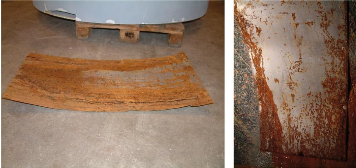
Figure 4-8. Drip shield attached to the demonstration drift at Äspö (right) and after detachment on the floor (left). Photos by H. Wimelius.
