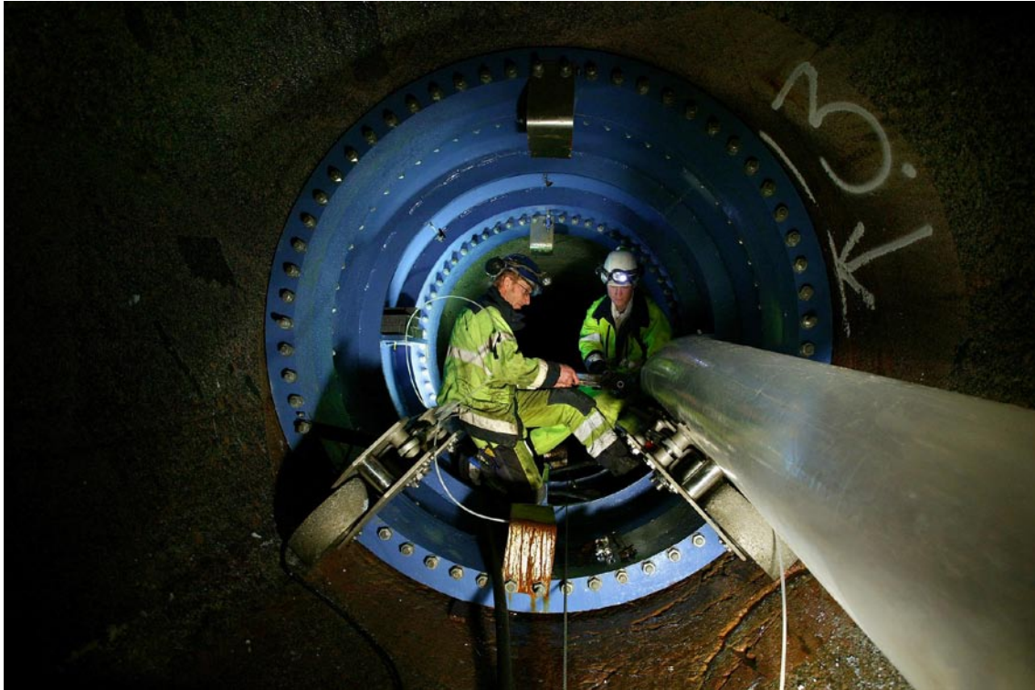
Figure 9-10. Mega-Packer in the drift with the personal working inside. Photo by Curt-Robert Lindqvist.
