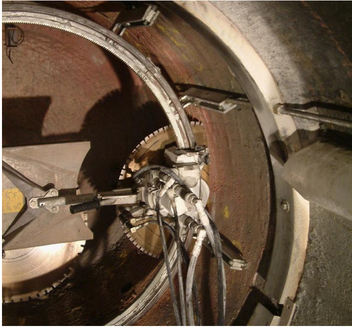
Figure 4-18. Sawing of a notch for the compartment plug by a specially developed rig.
