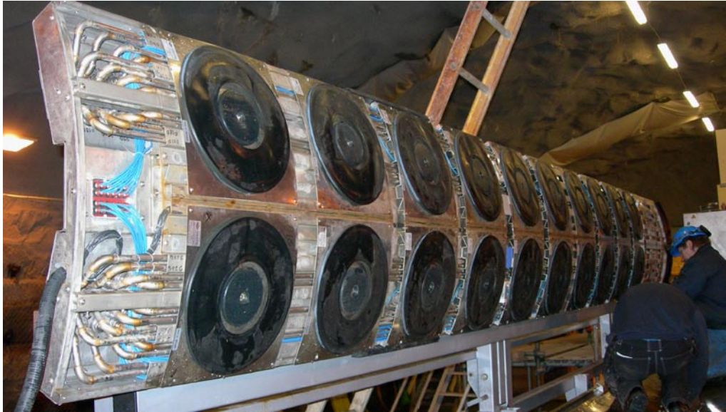
Figure 8-1. View of underside of the lift pallet during installation of water cushions.
