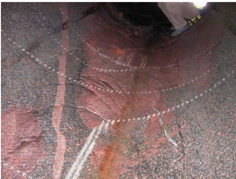
Figure 4-47. Some typical types of surface unevenness in deposition drift: rifle type grooves on the drift wall (top) and notches at fracture intersections on the floor (above). Note that some of the surface unevenness are due to rock fractures and not related to the excavation method.
