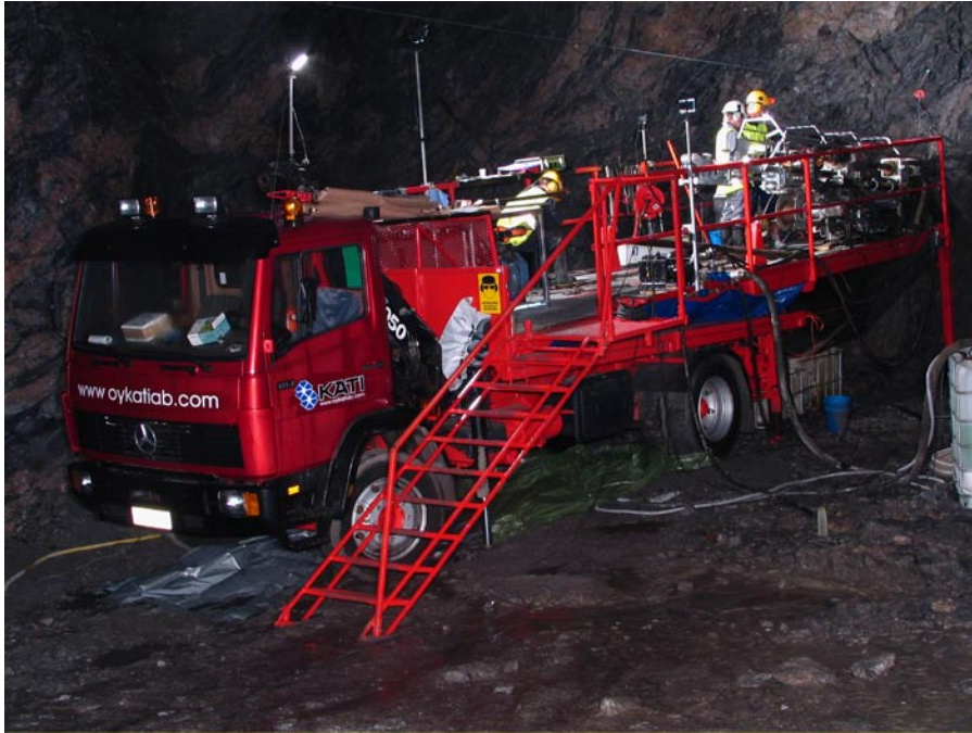
Figure 4-51. In ONKALO the drill rig installed on a truck has been used to core drill up to 200 m long investigation holes along the planned access tunnel.
