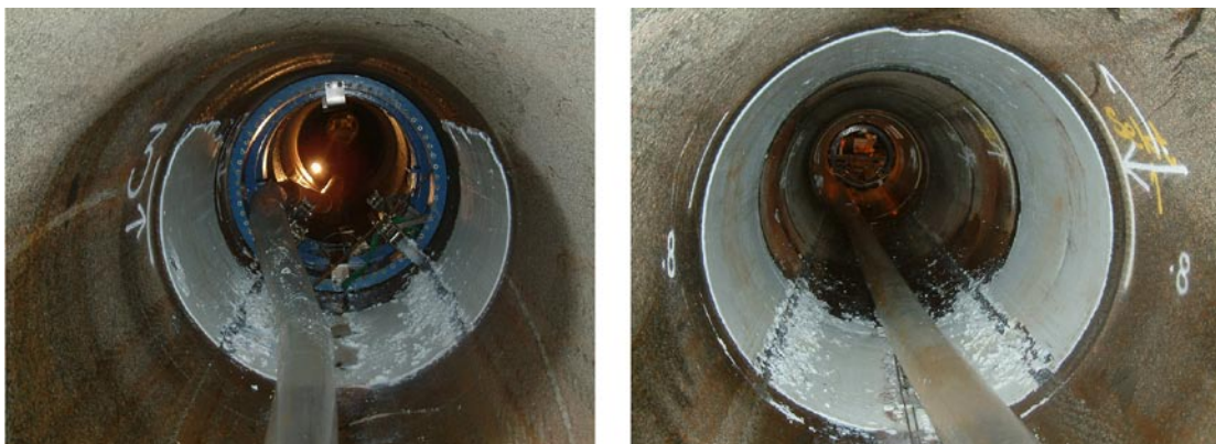
Figure 9-11. Two photos showing the grouted sections after removing the Mega-Packer. Left: Incomplete filling in Position 3. Right: Complete filling in Position 1. Photos by Linda Lindström, Magnus Kronberg.
