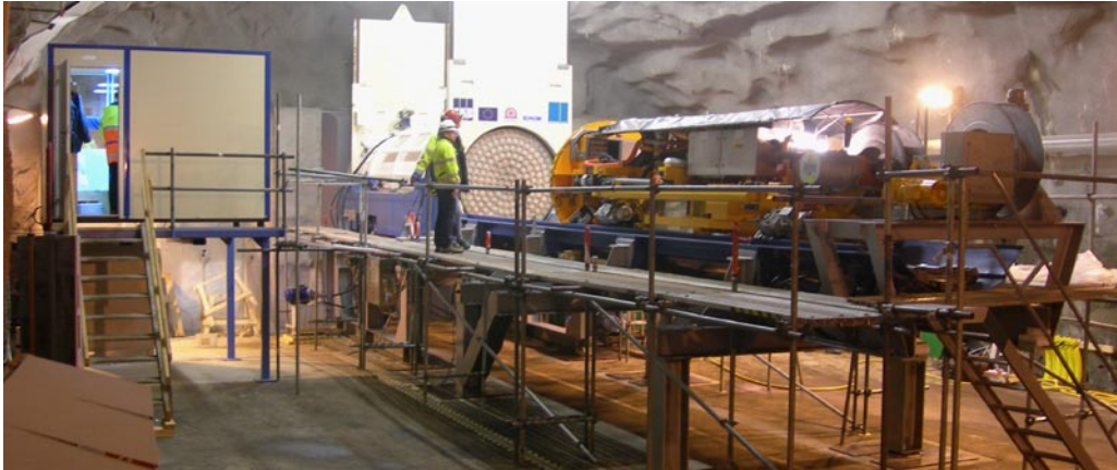
Figure 8-5. Set-up of equipment at the test site at Äspö HRL, level -220 m.
