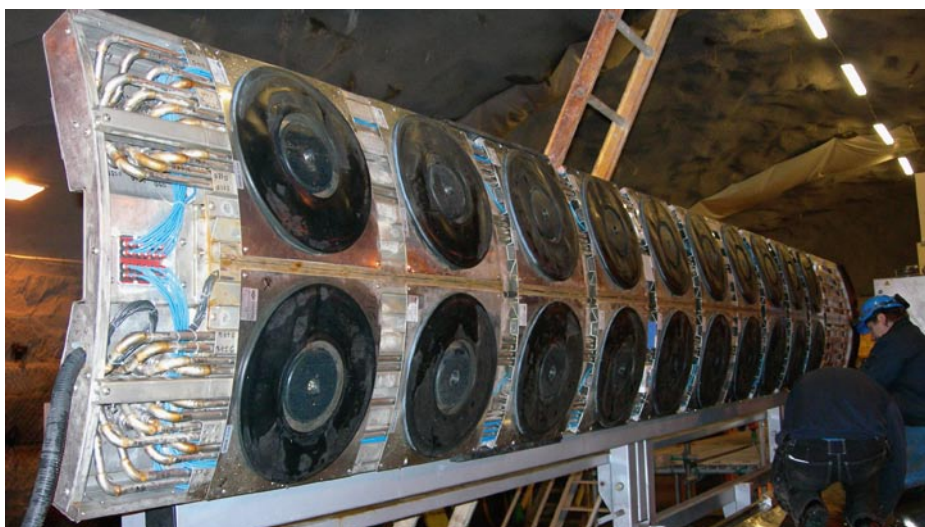
Figure 6-7. View of underside of the lift pallet during the installation of water cushions.
