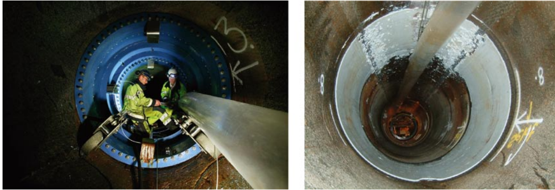
Figure 4-18. Left: Installation of the Mega-Packer in the Äspö HRL KBS-3H drift. Right: After grouting the Silica Sol is shown as a white rim at the drift periphery. The rim is later cleaned away.
