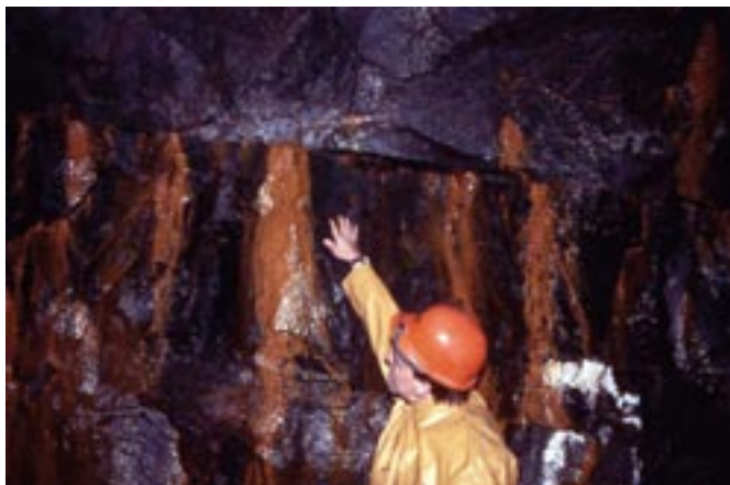
Figure B-1. Possible in-plane flow channels observed in the Bolmen tunnel as indicated by iron oxide precipitates at in-flow locations. Image taken from /Neretnieks 2006a/.
